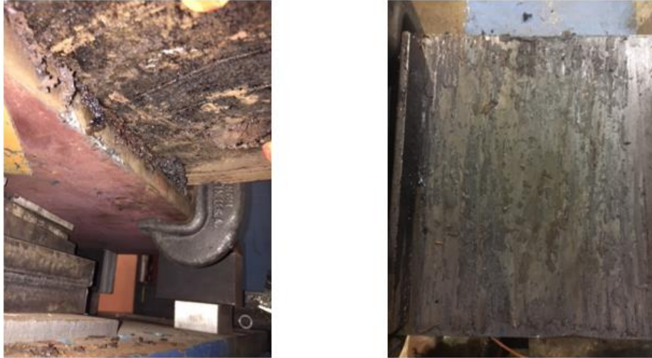
Figure 4-10: Creosote between tie and girder (left) and creosote on girder after testing on SP2 (right)
