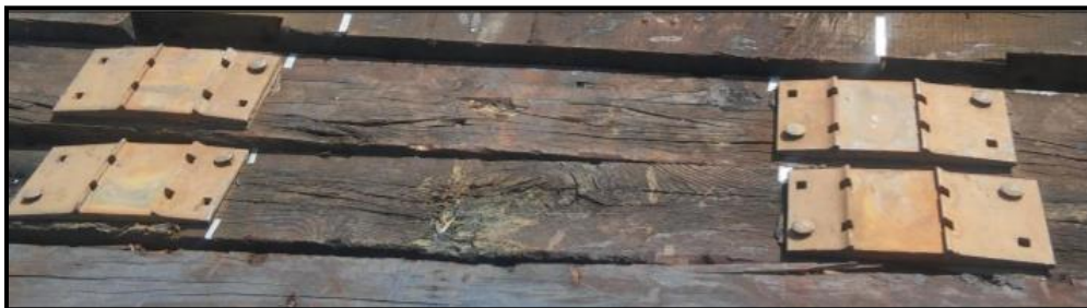
Figure 3-7: Tie plates, bearing pads, and railroad spikes on top of tie (Vasudevan, 2018)
