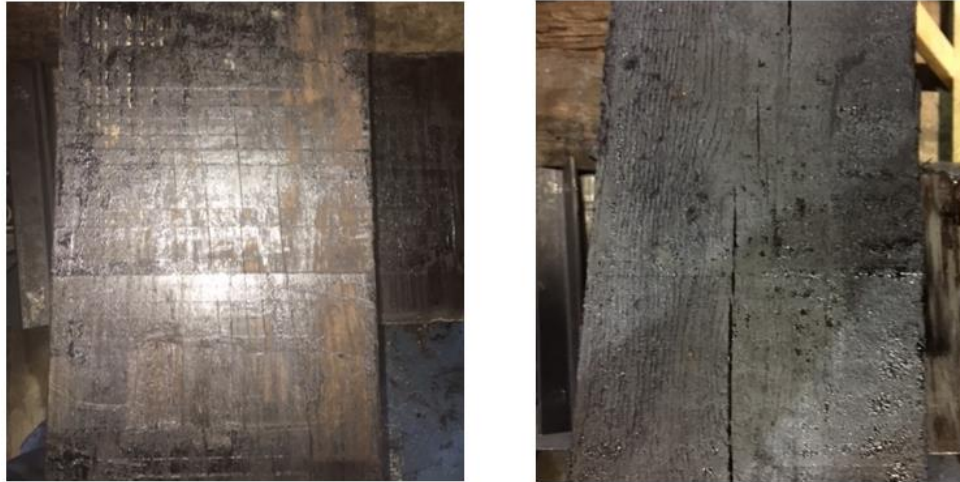
Figure 4-13: Side of O2 with low creosote retention (left) vs. side with high creosote retention (right)
