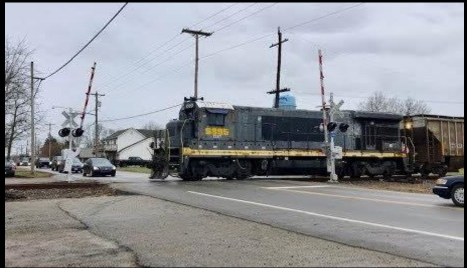
Inoperable Gates and Lights
