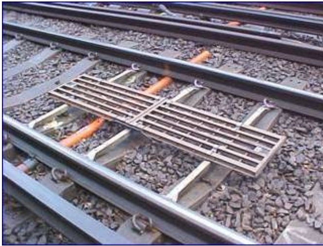
Figure 9: A pair of TPWS loops fixed to the track close to a signal. The two loops act as a tripping activator if a train attempts to run past a signal showing a stop aspect. Most main line signals in the UK are fitted with this system. There will also be two further loops on the approach to the signal set to match the required train approach speed. Photo: Author's Collection.
