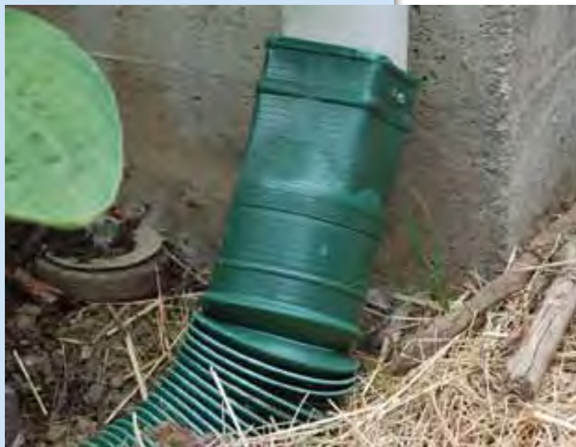
Figure 14. Downspout connected to downspout extension that directs flow away from a building's foundation. Note sheet-metal screws. (Photo: Robert Emanuel, OSU)
