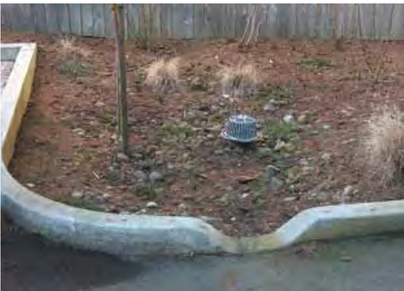
Figure 15: Curb-cut inlet for a parking lot and an overflow device (pipe and screen) for a parking lot in Gresham, Oregon. (Photo: Derek Godwin, OSU)
