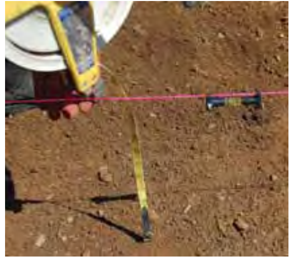
Figure 20: Using a combination of a line level and a measuring tape allows you to grade the base of the garden so that water will not pool in a particular location but will spread across the entire surface as evenly as possible. (Photo: Robert Emanuel, OSU)
