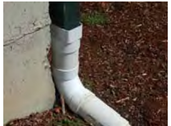
Figure 21: Four-inch ABS storm-drain pipe connects smoothly to a downspout from a roof to a rain garden in Pacific City, Oregon. (Photo: Robert Emanuel, OSU)
