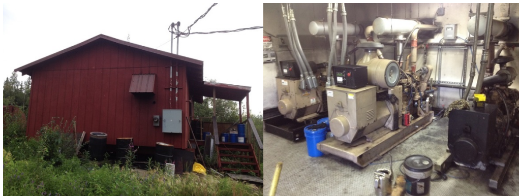
Figure 7. Rampart powerhouse (left) and generators (right)
