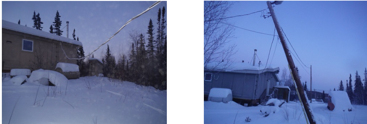
Figure 8. Rampart distribution lines (left) and leaning power poles (right)
