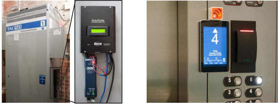
Figure 9. Elevator instrumented in the machine room with an electric meter and DAQ server (Left) and in the cab with a FRESH node and Android tablet (Right) to implement an Elevator Energy Display (EED).
