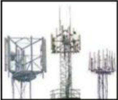
~2,000 installed telecom systems
