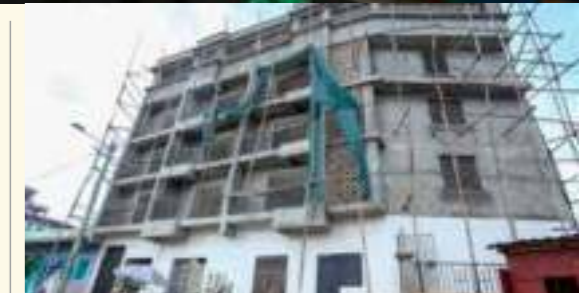
Ongoing construction of the guest house owned by Fatuma Nur Mumin, a business owner in Moyale Town.
