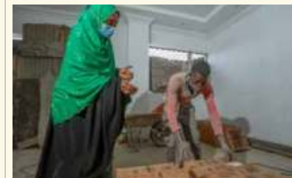
Mumin with a construction worker at the guest house being build in Moyale Town.
