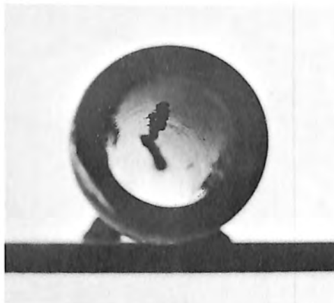
Figure 29. Interior of PVC pipe showing residue of material removed during mechanical drilling. Photo P801D-74395NA
