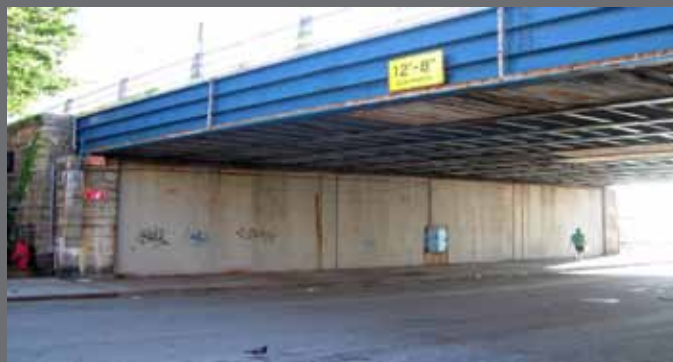
Existing Substandard Condition of Bay Ridge Avenue Bridge
