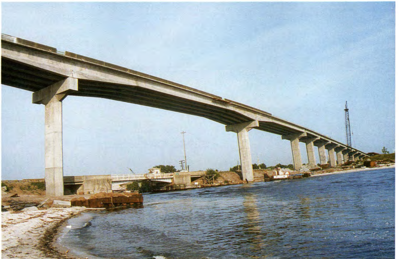
Fig. 2. Partial view of Highland View Bridge showing 250 ft (76.2 m) main span in foreground.
