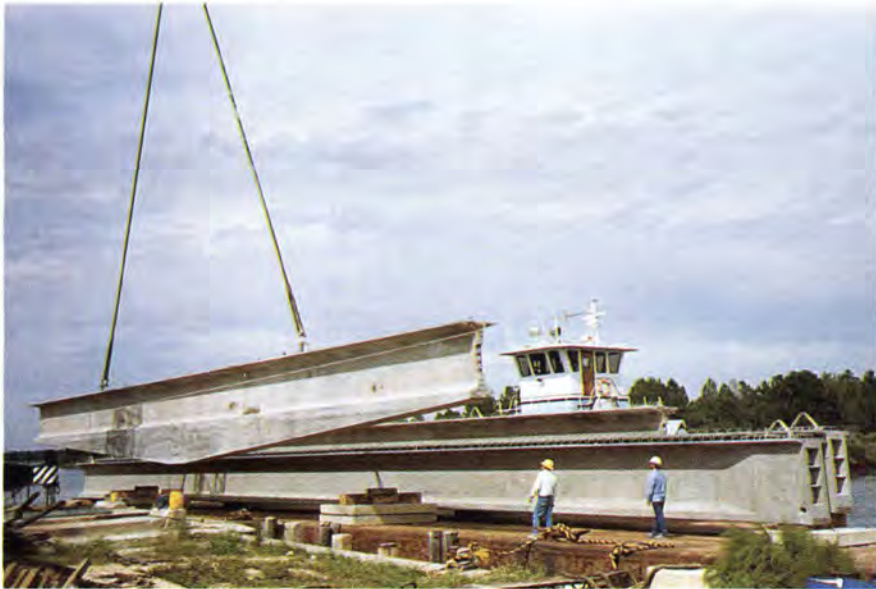
Fig. 9. After arrival at the bridge site, a haunched girder section is lowered by crane for temporary storage.
