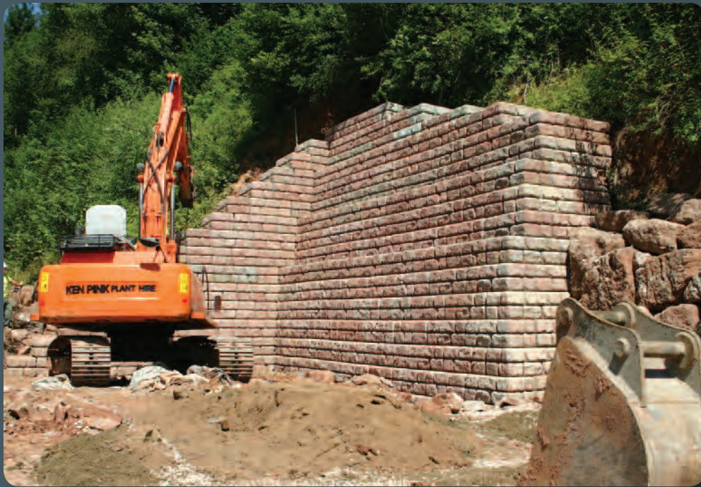
9mt tall wall protecting against rock fall - coloured to match local stone
