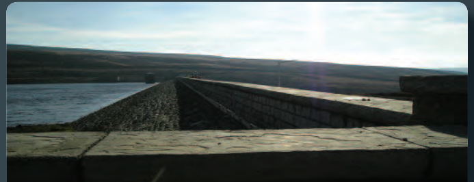
Wavewall on Yorkshire Water reservoir
