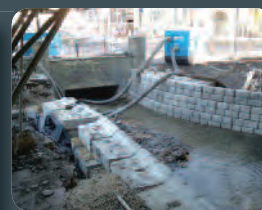
Erosion control of an underground stream. Listed building saved, wall took 3 men 17 days.
