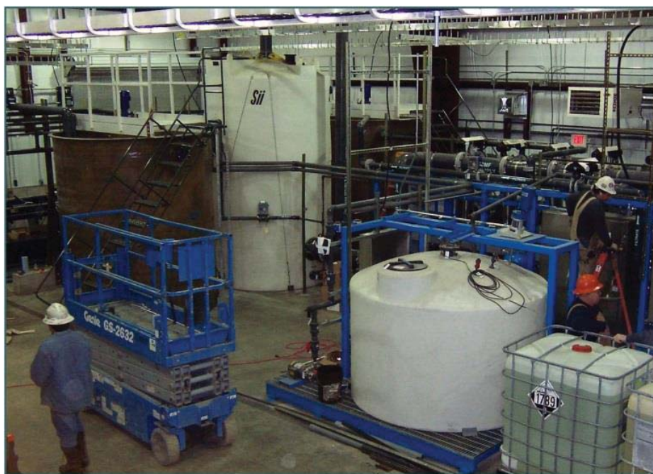
Figure 21: Ceramic Microfiltration System at the Upper Blackfoot Mining Complex, Montana
