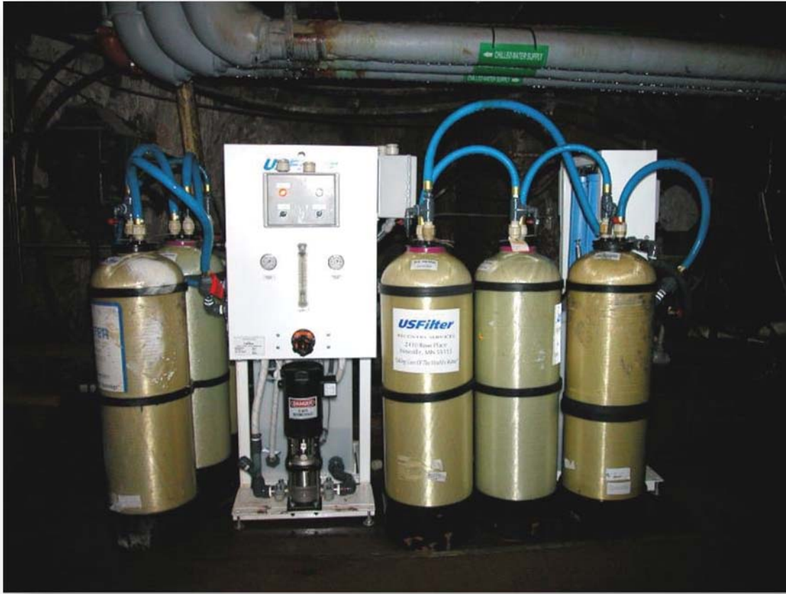
Figure 19: In-Mine Ion Exchange Treatment System at the Soudan Mine
