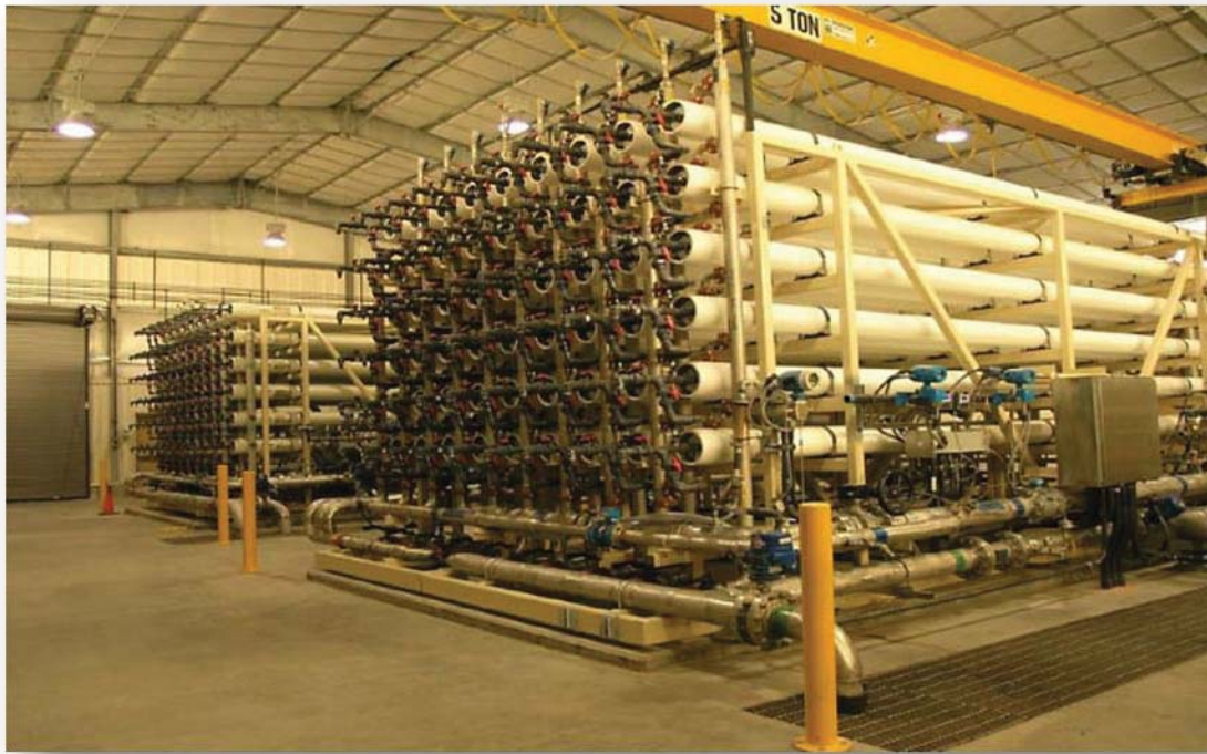
Figure 12: Two Reverse Osmosis Treatment Racks at the BCWTP
