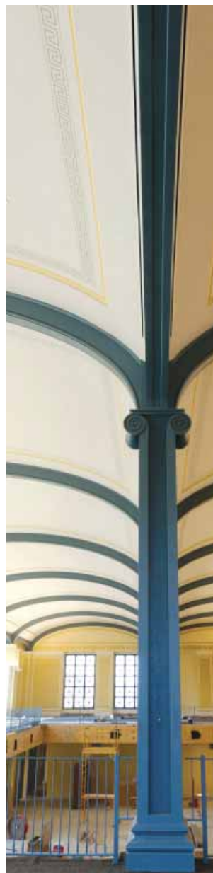
4 Bronx Community College's, 98,000 sq. ft. North Instructional Building and Library, provides classrooms, a library, a café, a two-story commons, study rooms and lounges.
