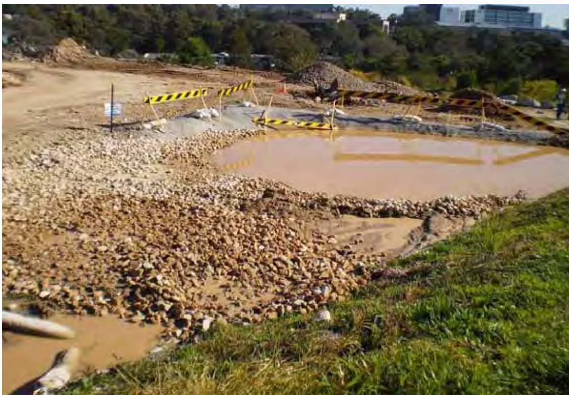
Photo 66 - Sediment basin for wash bay facing north
