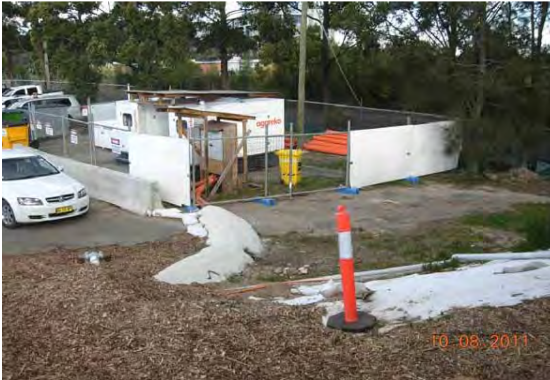
Photo 29 - Deisel-powered generators and associated tank near south-west corner of Leighton sheds
