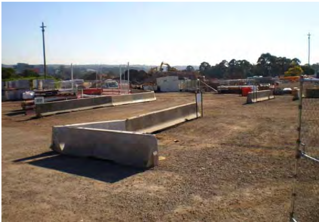
Photo 50 - Facing north towards stockpiles in centre of site from in front of site office shed area
