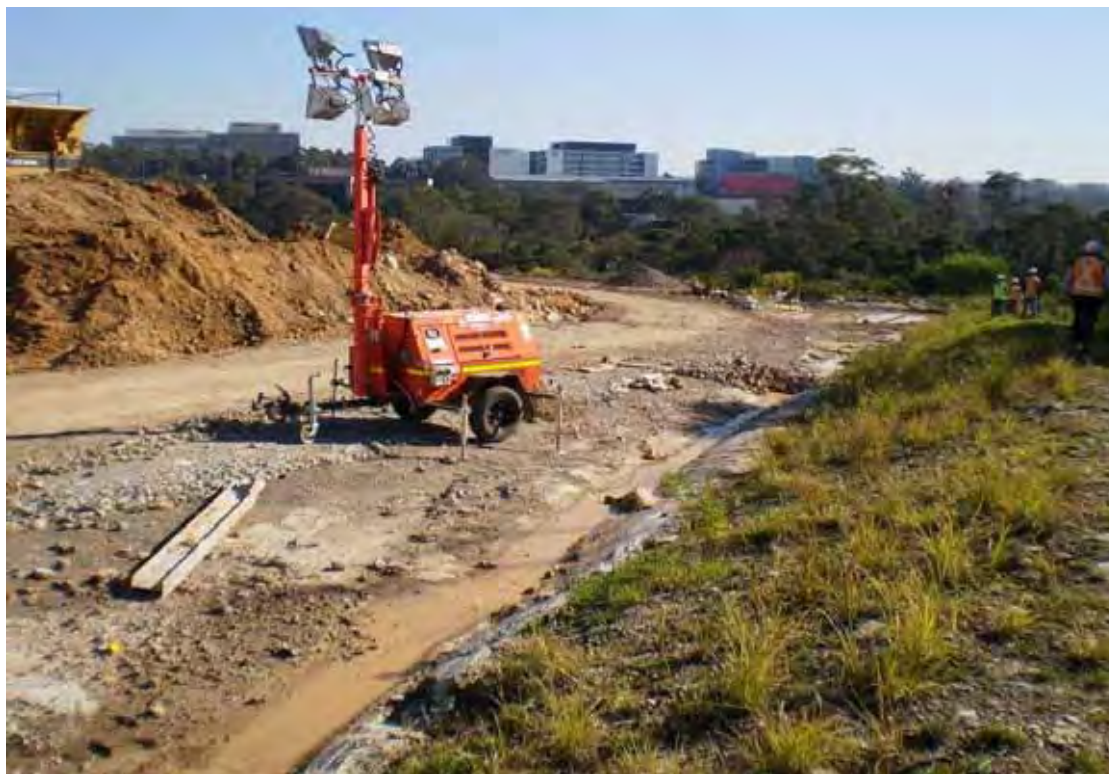
Photo 64 - Drainage of wash bay water towards sediment basin within northern portion of compound
