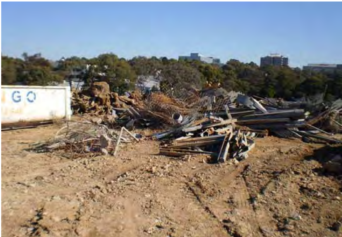
Photo 70 - Discarded metal located north of stockpiles facing north
