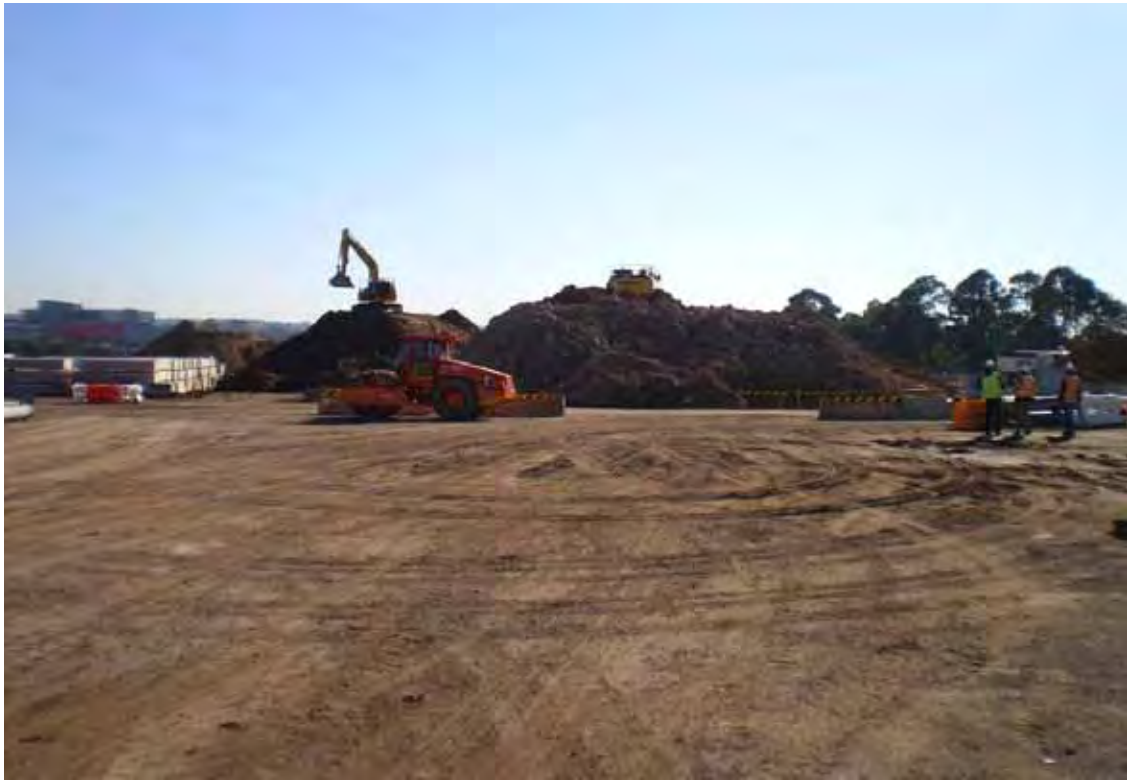
Photo 57 - Stockpiles generated from M2 Upgrade works taken from central portion of compound facing north
