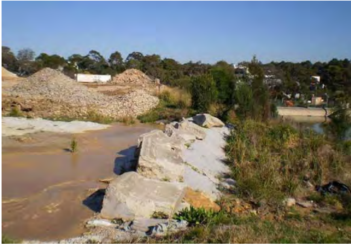
Photo 67 - Bunded sediment basin with large detention basin at northern extent of compound facing west
