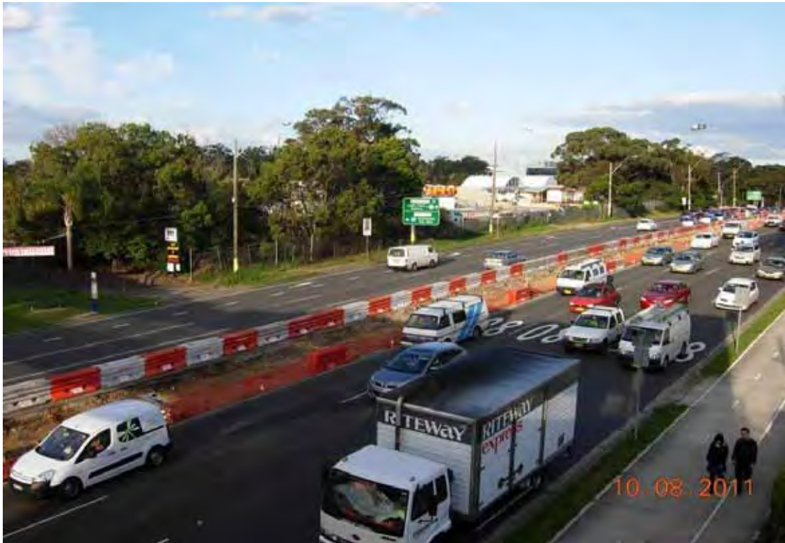
Photo 43 - South-western boundary of site facing south-east from pedestrian bridge across Epping Road
