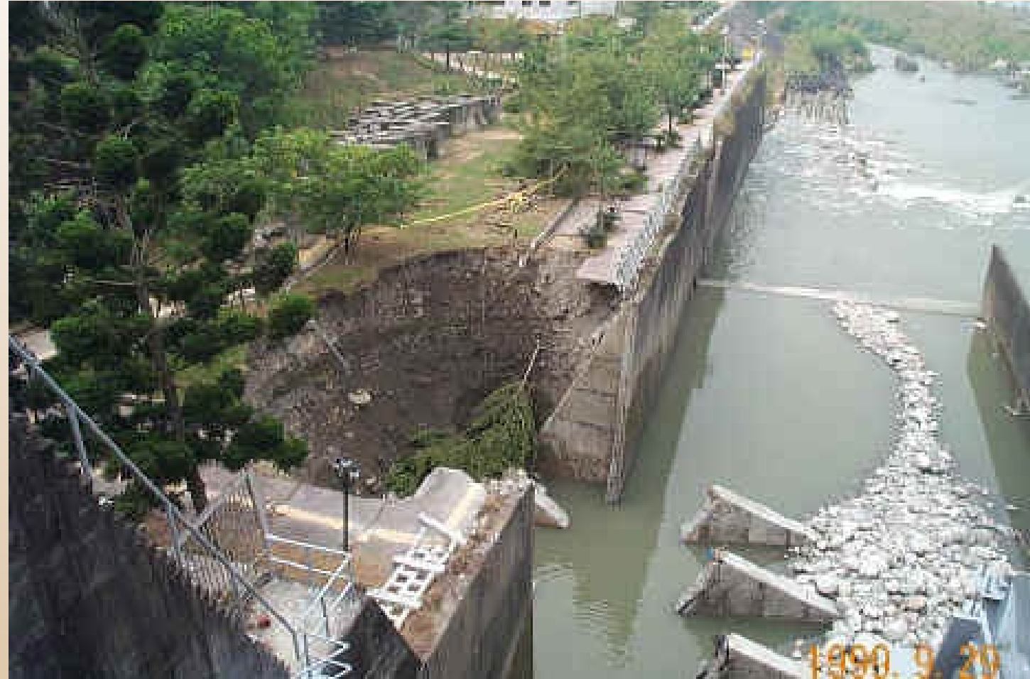
Shi-Kang Dam - 1999 Chi-Chi, Taiwan Earthquake – immediate aftermath
