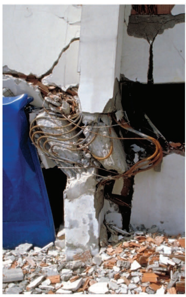
1999 Kocaeli, Turkey Earthquake
