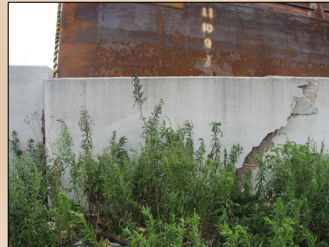
Damage to Floodwall by an Aberrant Barge During Hurricane Gustav (Orleans East Parish)
