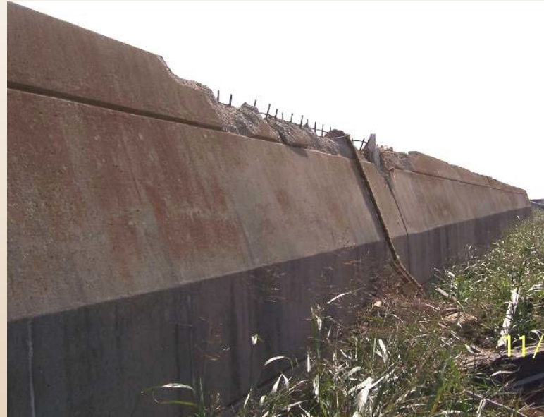
St. Bernard Parish, New Orleans - Damage to top of I- Wall from a Barge: 2005 Hurricane Katrina
