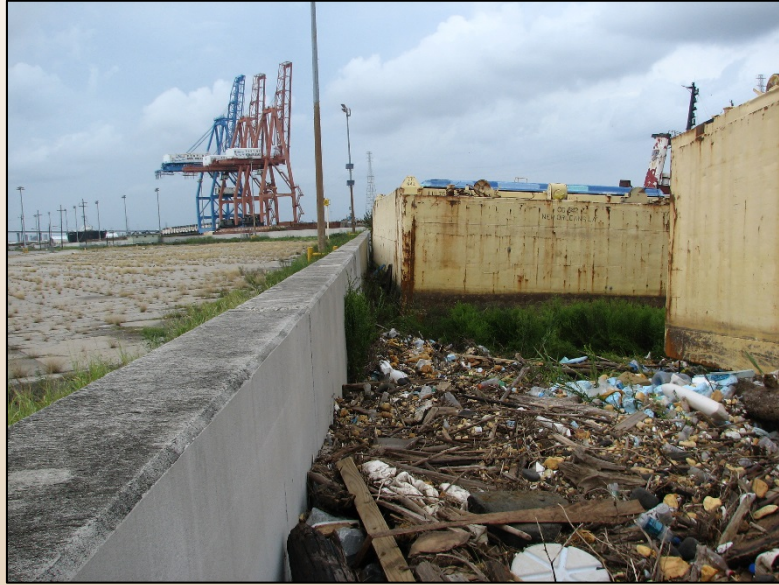
New Orleans Floodwall: Barges against face of floodwall 2005 Katrina
