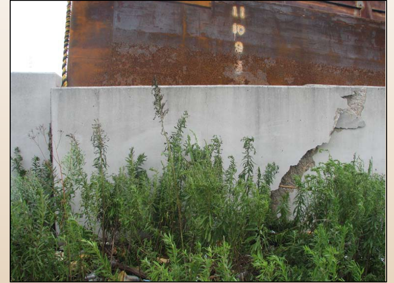
Damage to Floodwall by an Aberrant Barge during Hurricane Gustav, 2008 (Orleans East Parish)
