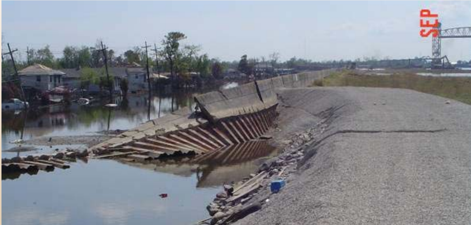
New Orleans Lower Ninth Ward Failed I-Wall: September 2005 Hurricane Katrina
