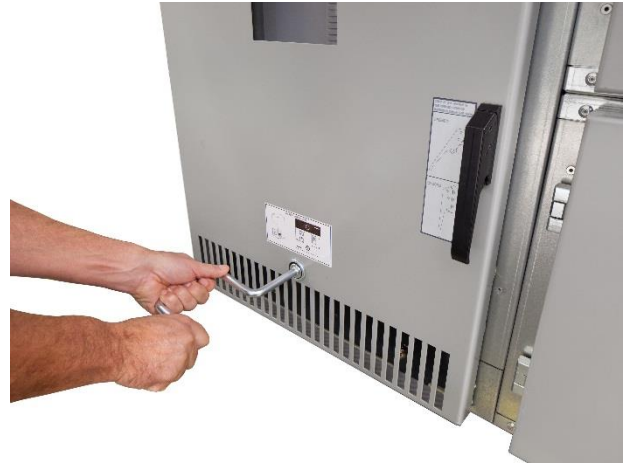
Figure 23: Racking tool inserted into racking port
