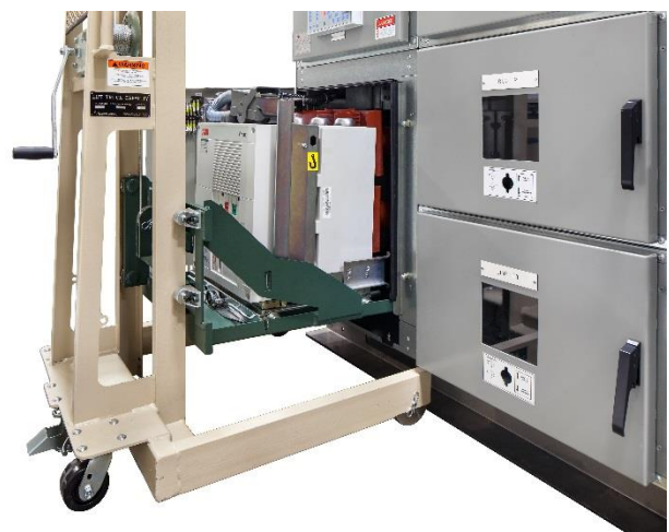
Figure 17: Lift truck holding Vmax/A
