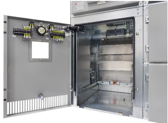
Figure 11: Breaker module with open door
