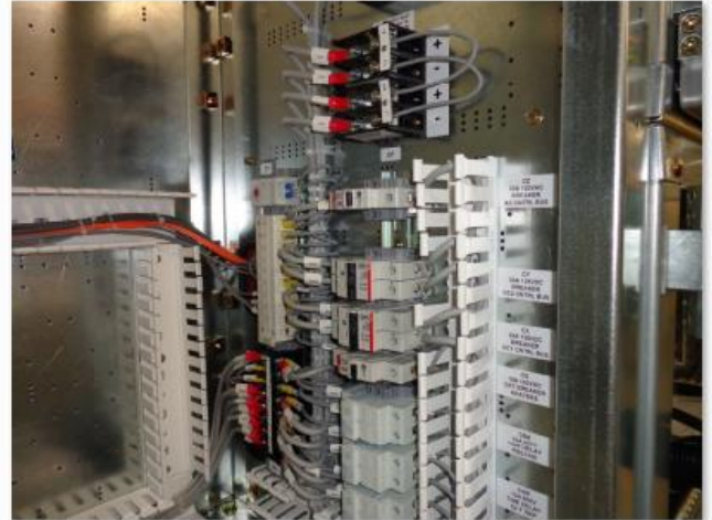
Figure 1: Heater load terminals in low voltage compartment
