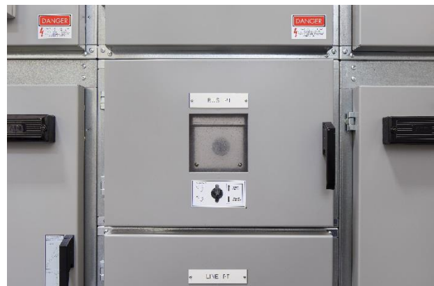
Figure 26: PT module door closed and element in disconnect position
