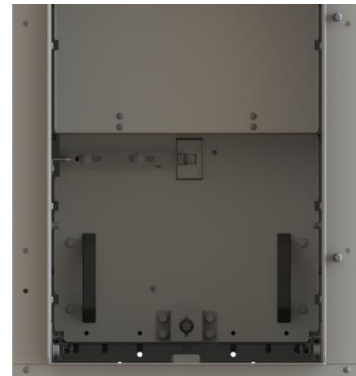
Figure 25: Front view of CPT compartment with secondary breaker interlock shown
