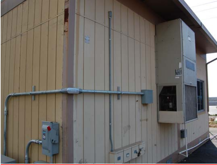
Building with original HVAC system 42WH1
