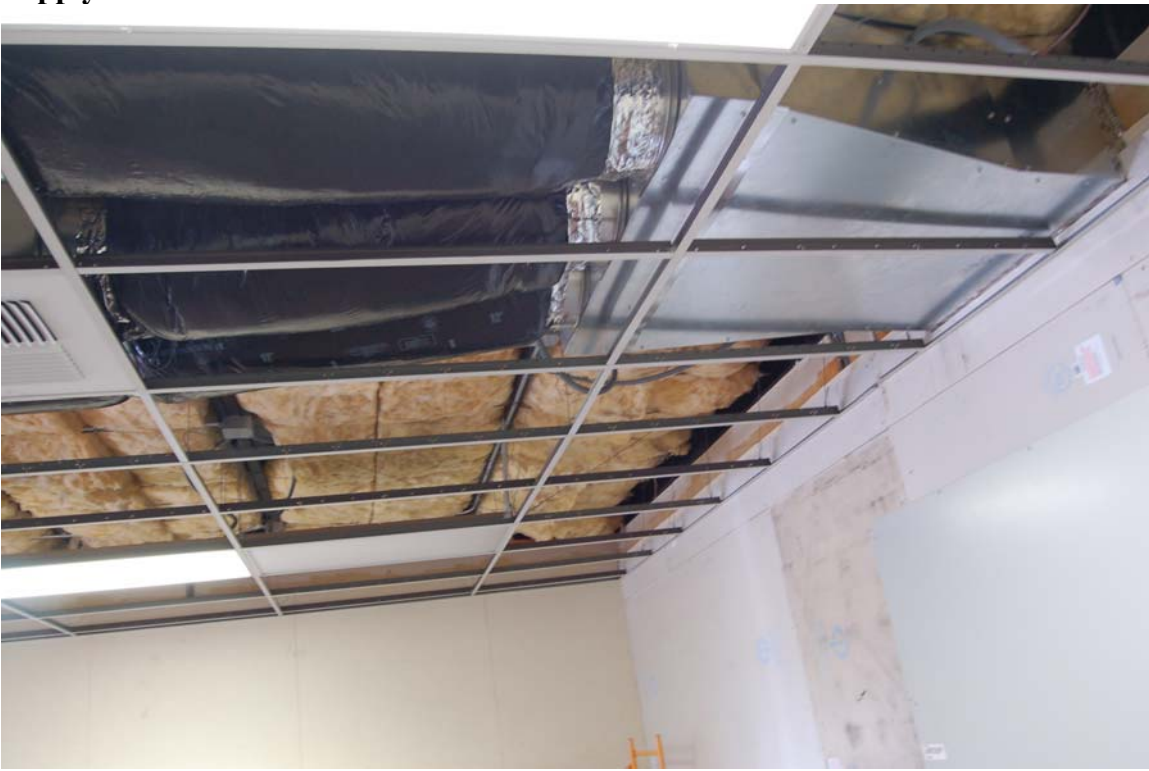
Supply Air Acoustical Plenum installed – 3 outlets.
