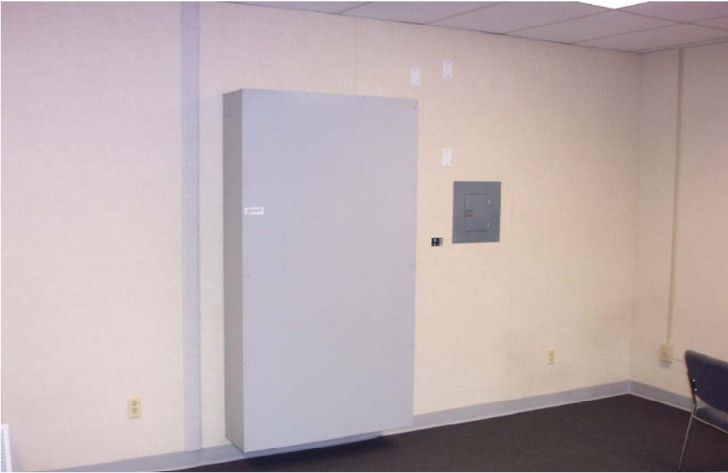
Indoor modular relocatable classroom view of Return Air Acoustical Plenum.
