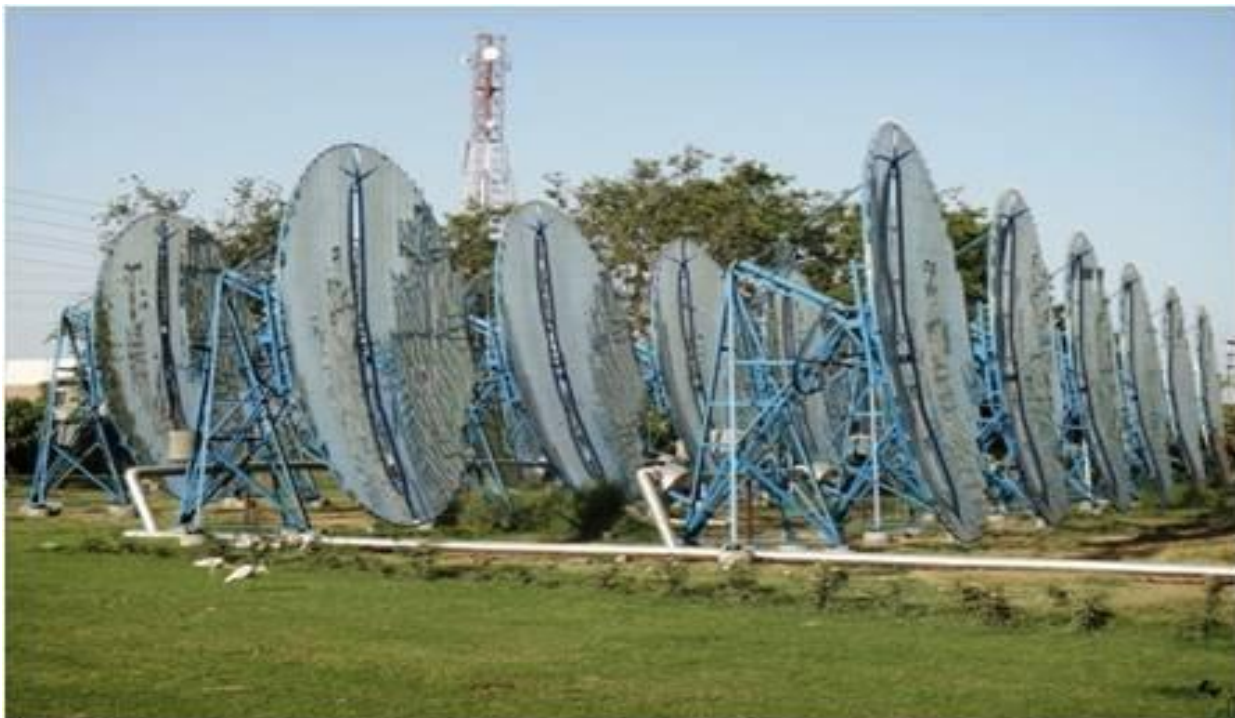
Figure 4: Solar Concentrating system installed at Resham Vibhag, Premnagar, Dehradun
