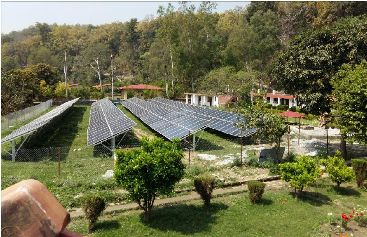
Figure 3: 500 KW Solar power plant at Ramnagar, Nainital
