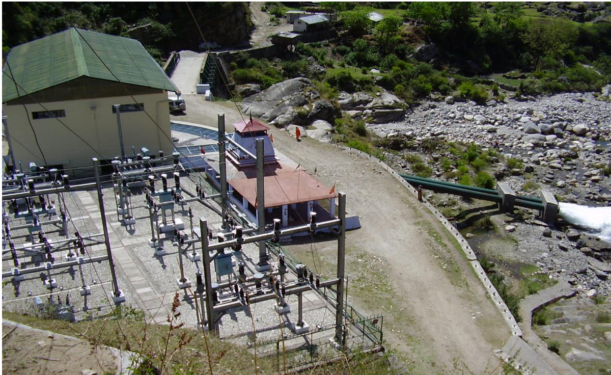
Figure 1: Pilangad Small Hydro Power Plant
