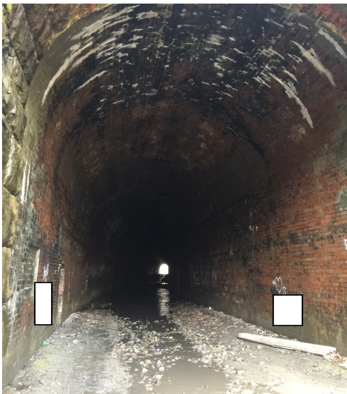
Interior of the Kingsville Tunnel looking west. Photo sanitized due to questionable graffiti. Photo by Janis Bland
