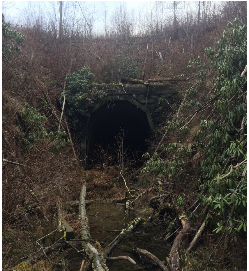
Orr Tunnel, east portal with framing timbers still in place. Photo by Janis Bland
