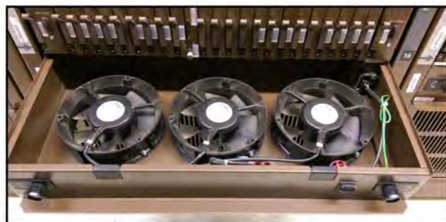
DMS-100 NTRX91AA FAN UNIT w/ EXISTING FANS
