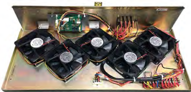
CONVERTED NORTEL DMS-100 NT3X90AC FAN TRAY * WITH (5) NEW 48V FANS & NEW ALARM CONTROL BOARD
