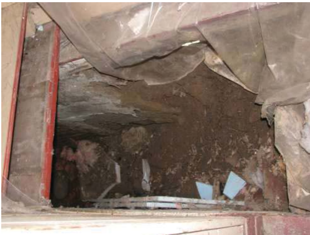
Plate 14: Collapsed stairway leading to basement under kitchen
