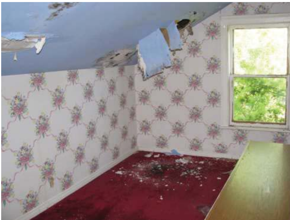
Plate 10: Upstairs bedroom with mould and ceiling damage
