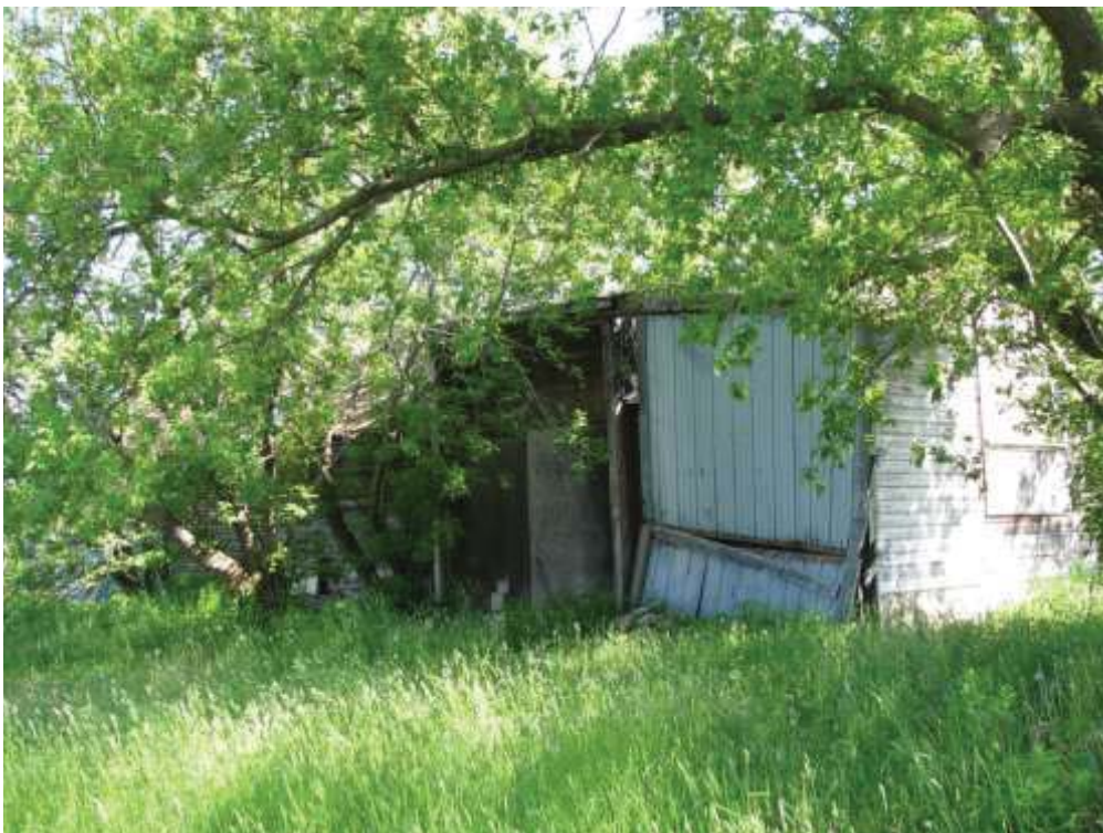
Plate 18: Wood frame shed supported by aluminum siding
