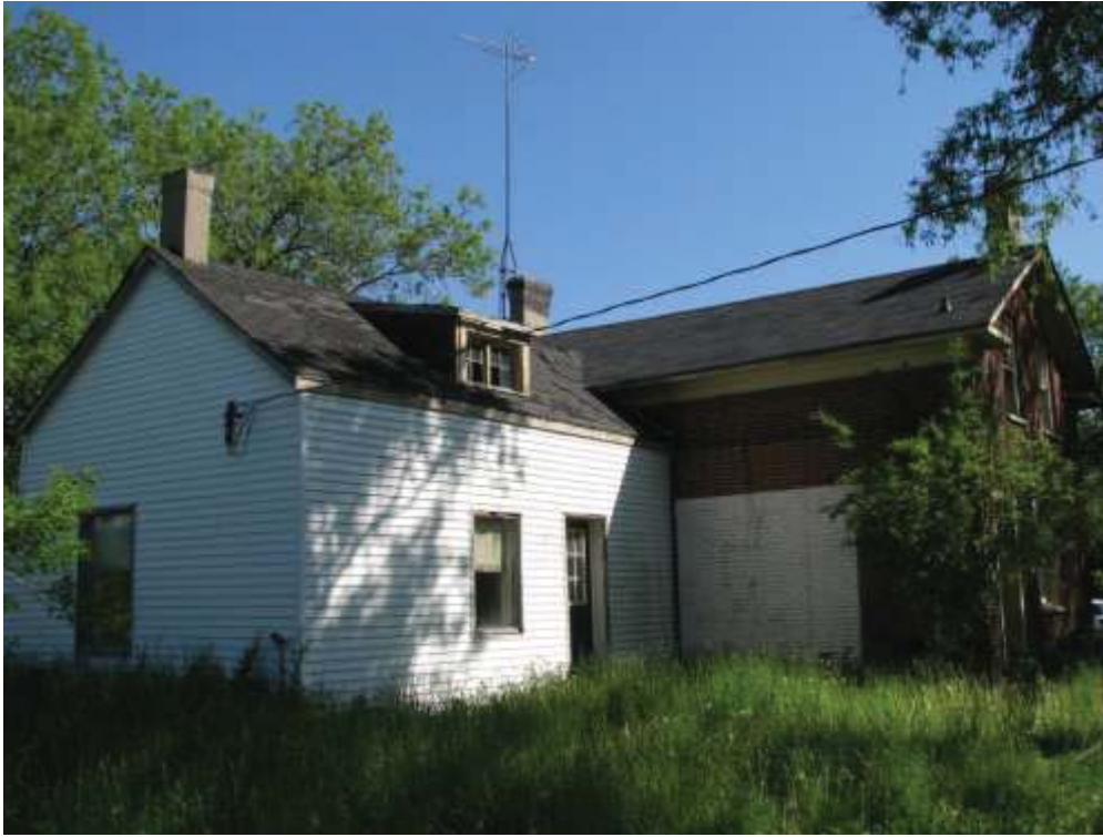
Plate 12: Kitchen addition with brick discolouration to right
