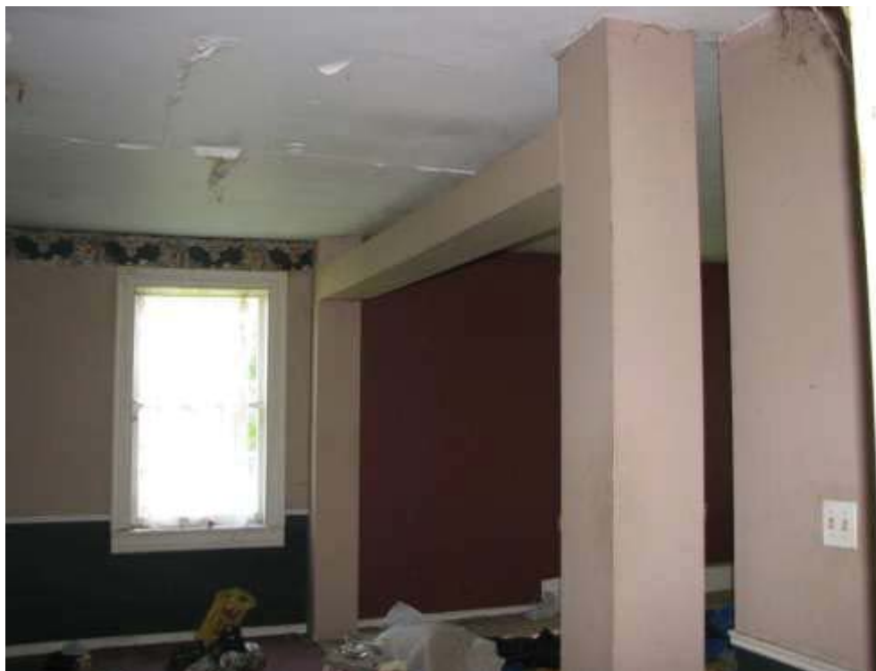
Plate 9: Interior of brick structure main floor with ceiling damage visible
