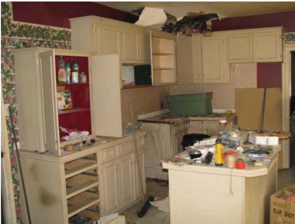
Plate 13: Downstairs kitchen with ceiling damage
