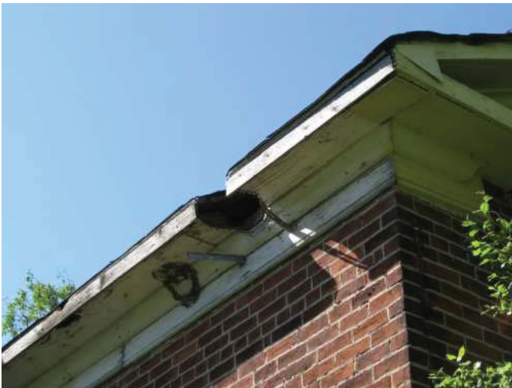
Plate 7: Detail of damage along roof edge
