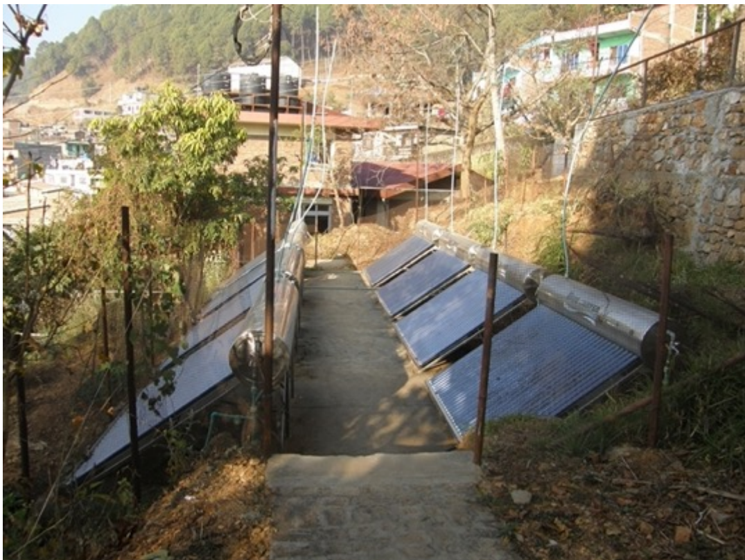
Solar water heaters
