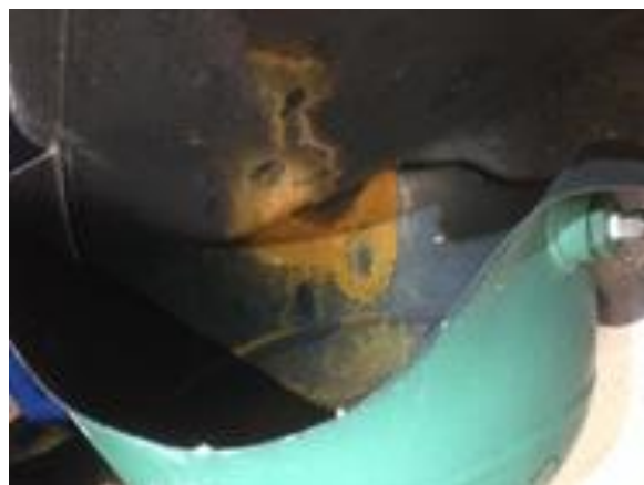
Figure 5: Rust inside the damaged gas storage tank as observed by the Investigative Team.
