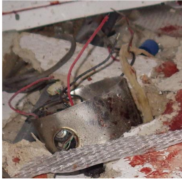
Figure 27: Pressure gauge housing as found by HFD
