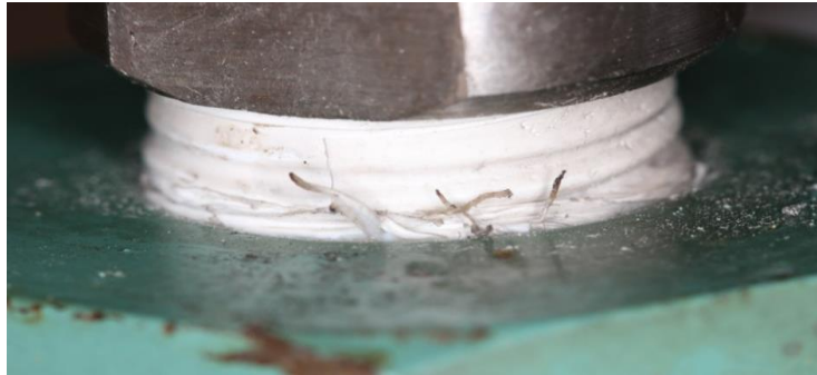
Figure 32: Photo of gauge stem Teflon tape that appears to be charred and melted.
