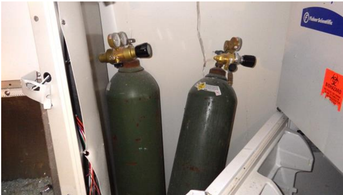
Figure 21: Oxygen cylinders used to fill the gas storage tank (standing upright) and used for the second postdoctoral researcher's ongoing experiment (tilted). The latter oxygen cylinder was open at the time of the explosion.
