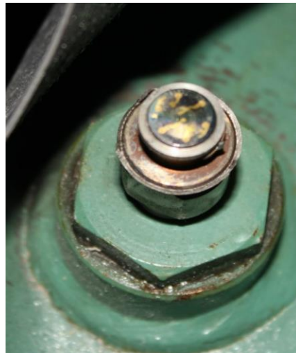
Figure 26: Pressure gauge diaphragm still attached to the threaded gauge stem that was still threaded into a bushing on the tank. On the external surface (non-wetted side) of the diaphragm one can see markings where the strain sensors were attached to the diaphragm.
