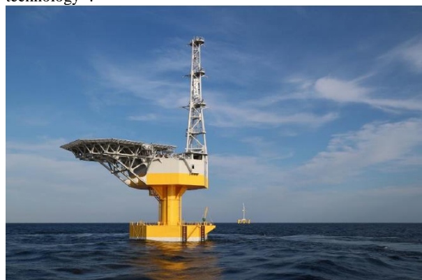
Fig. 2 Floating electrical substation off Fukushima. (picture courtesy of Japan Marine United )
