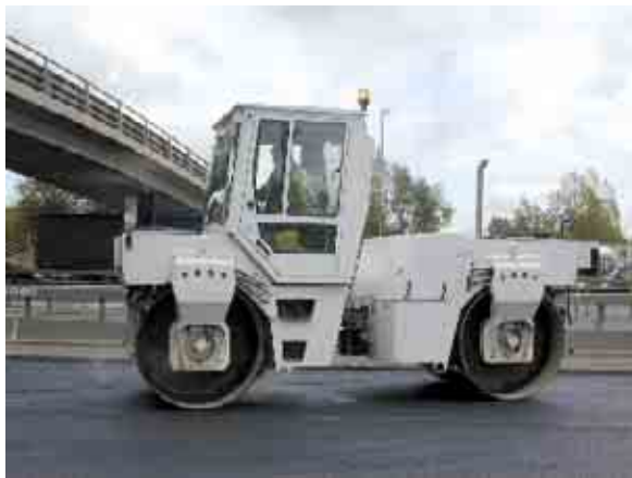
Figure A1.6.1 Bomag BW161 AD2 10-tonne articulated twin-drum vibrating roller compacting freshly-laid hot asphalt on M25
