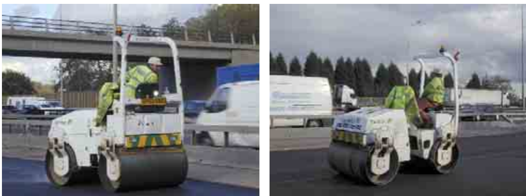
Figure A1.7.1 Bomag BW138 AD 4-tonne articulated twin-drum vibrating roller finishing partially-compacted hot asphalt on M25
