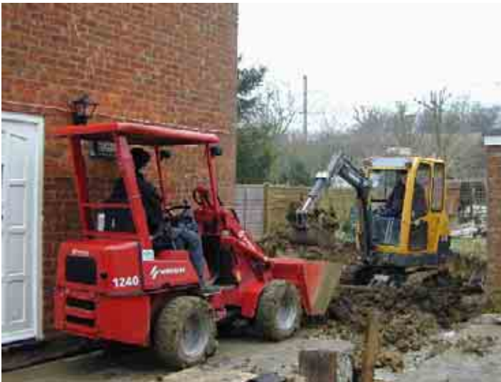
Figure A1.13.1 Volvo EC15B 1.5 tonne compact 360° excavator excavating footings for house extension and patio
