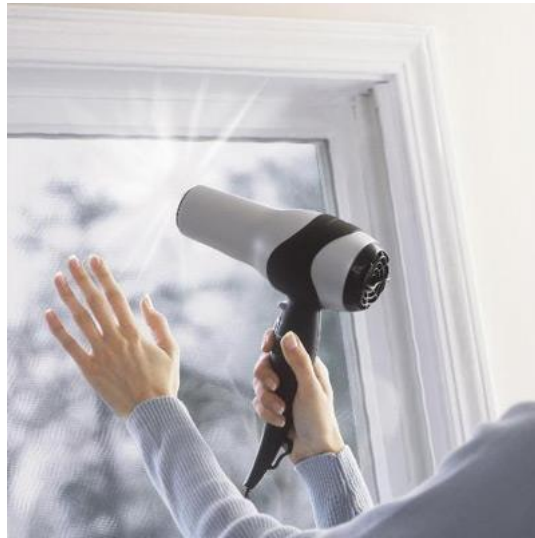
Figure 83: DIY installation of plastic around window frame. Image Source: This Old House, 2013
