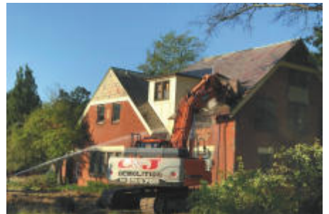
County funds will cover costs to finish the demolition project at Parmadale.
