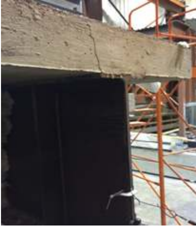
(a) Crack at end side of composite beam (CB3)
