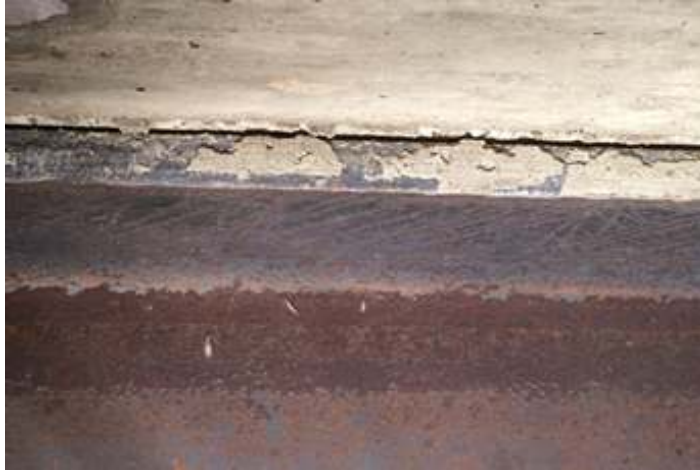
(b) Separation of concrete slab (CB4)
