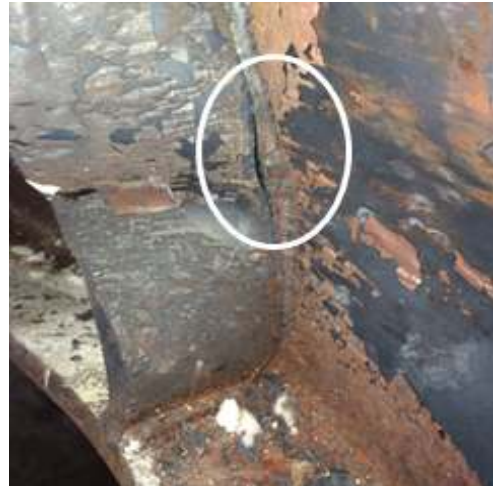
(b) Rupture of weld in stiffener
