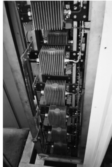
Figure 4: Dual Power Rectifier Bridge Assembly located in the Generator Auxiliary Compartment
