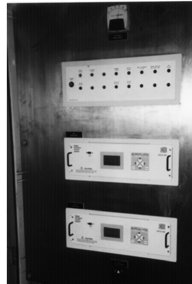
Figure 10: Dual digital control modules with automatic transfer and a local alarm/status LED
