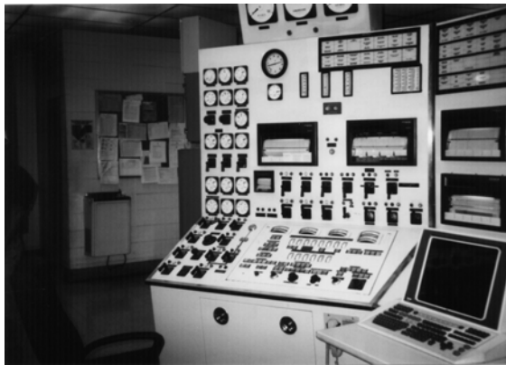
Figure 11: Existing generator controls and metering located at the BTG control panel are interfaced to the new digital control system
