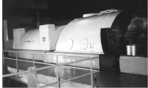
Figure 1: Main field-excited steam turbine generator
