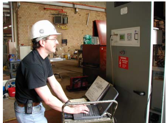
Figure 14: Start-up and commissioning of the new digital voltage regulator system is easier with all adjustments for setting the generator response, limits, protection, etc. at your fingertips via the serial port connection to your laptop computer.
