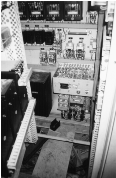
Figure 7: Voltage regulator and exciter field rheostat in the excitation switchgear lineup for a 40MVA steam turbine-generator
