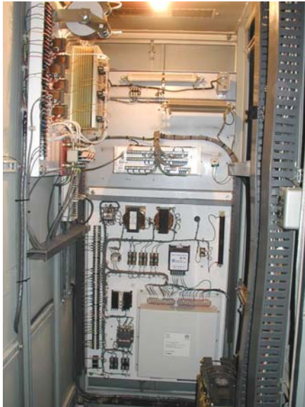
Figure 13: Retrofit of a new digital voltage regulator system into SCT-PPT excitation switchgear lineup
