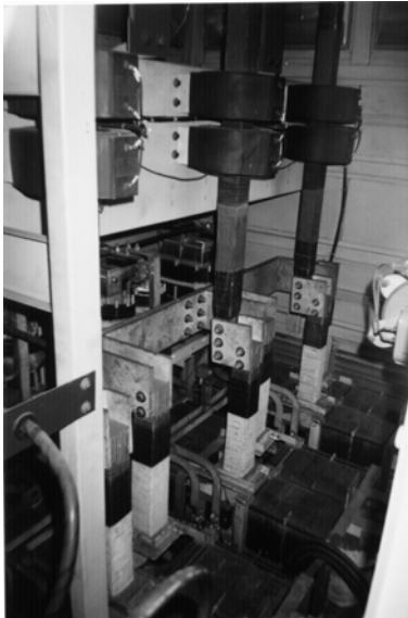
Figure 2: SCTs and linear reactors located on the Generator Neutral Bus
