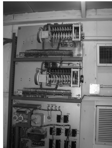
Figure 8: Motor operated pot for AC and DC voltage regulator
