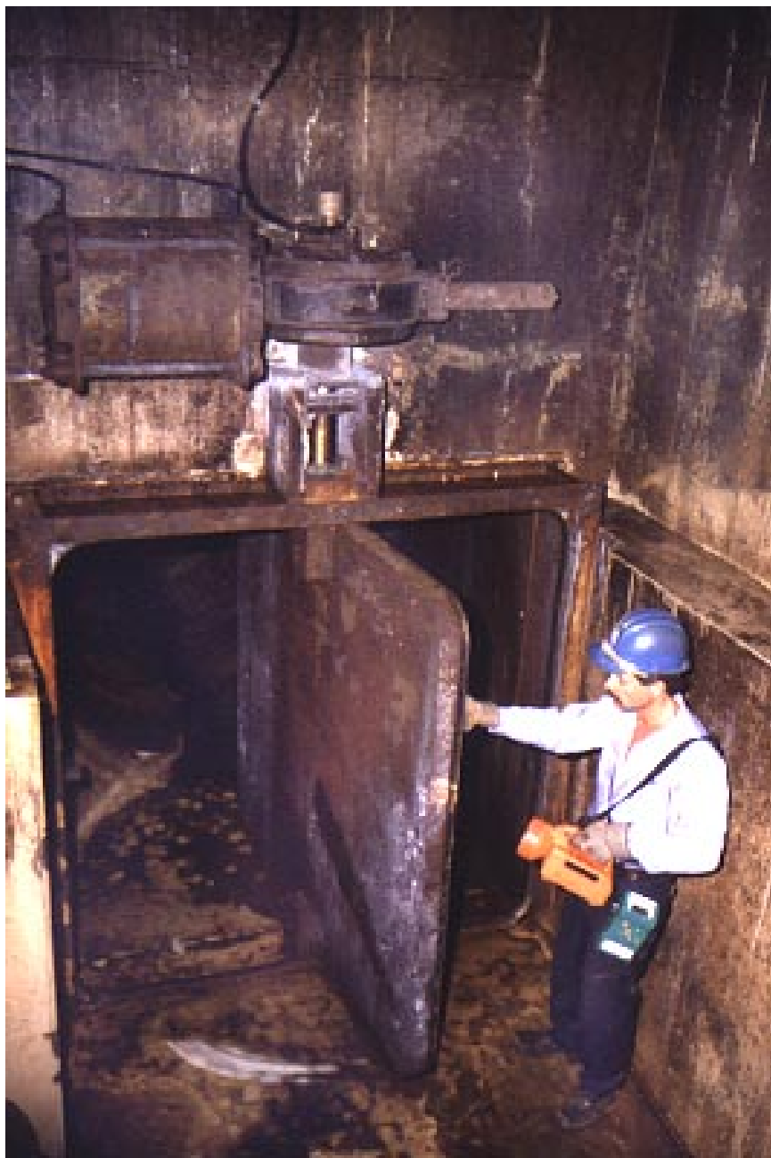
Many valves are located in hostile, hard-to-reach environments. By automating them, several benefits result, including less risk of worker injury, increased productivity, and improved efficiency. Here, a P Range pneumatic actuator is used to operate a large butterfly valve in a tunnel.
