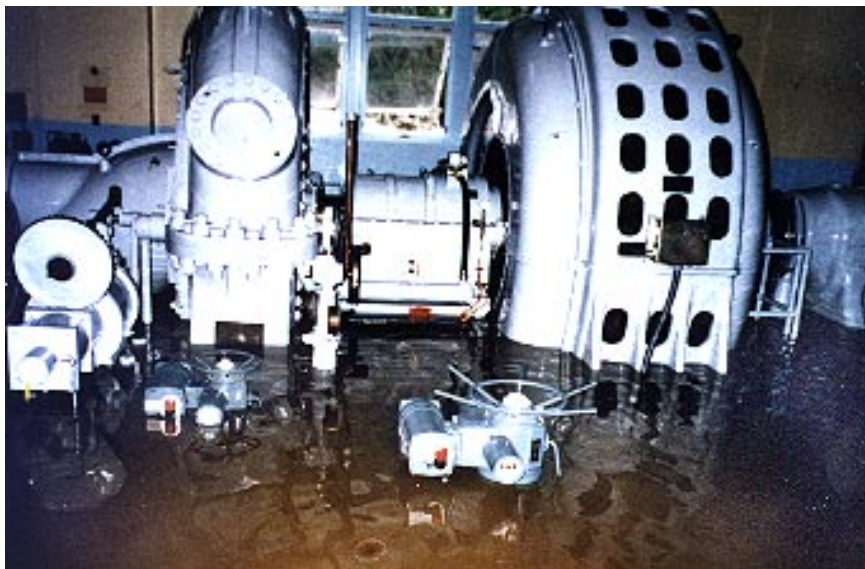
When a disastrous flood inundated the Tacoma Public Utilities' La Grande hydro plant on the Nisqually River in Washington, the Rotork actuators pictured above "were as good as new," according to Bill Jones project manager for the Nisqually Hydro Project.
