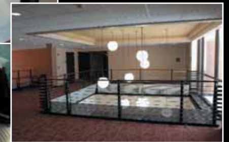
Engineering the changes required to open up the entry into the second floor to create an atrium with added glass presented a distinct design challenge.
