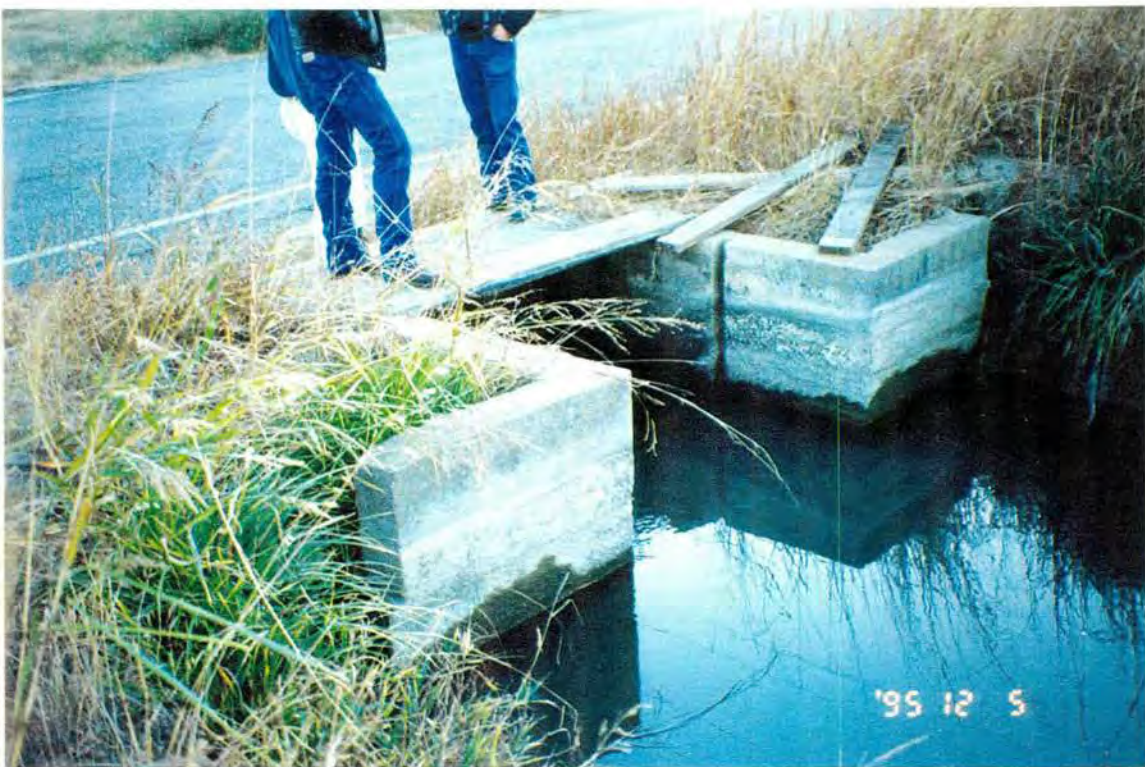
Photograph 14. - Turnout site from a lateral canal to a sublateral. Possible site for a motorized gate to control flow distribution in a lateral/sublateral distribution system.
