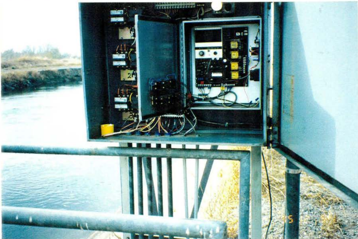
Photograph 6. - Control unit (Sierra Controls) at Walker check. Still automatically controls upstream water level.
