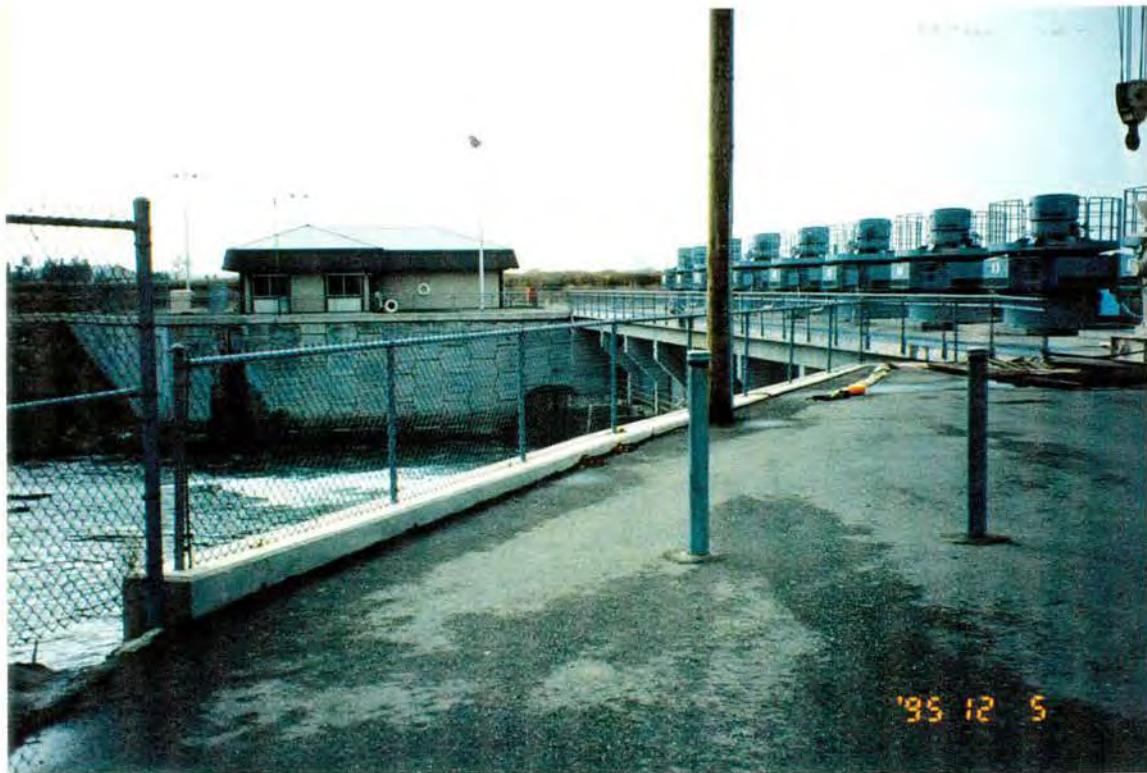
Photograph 11. - Glenn Colusa canal - main pumping plant on the Sacramento River.
