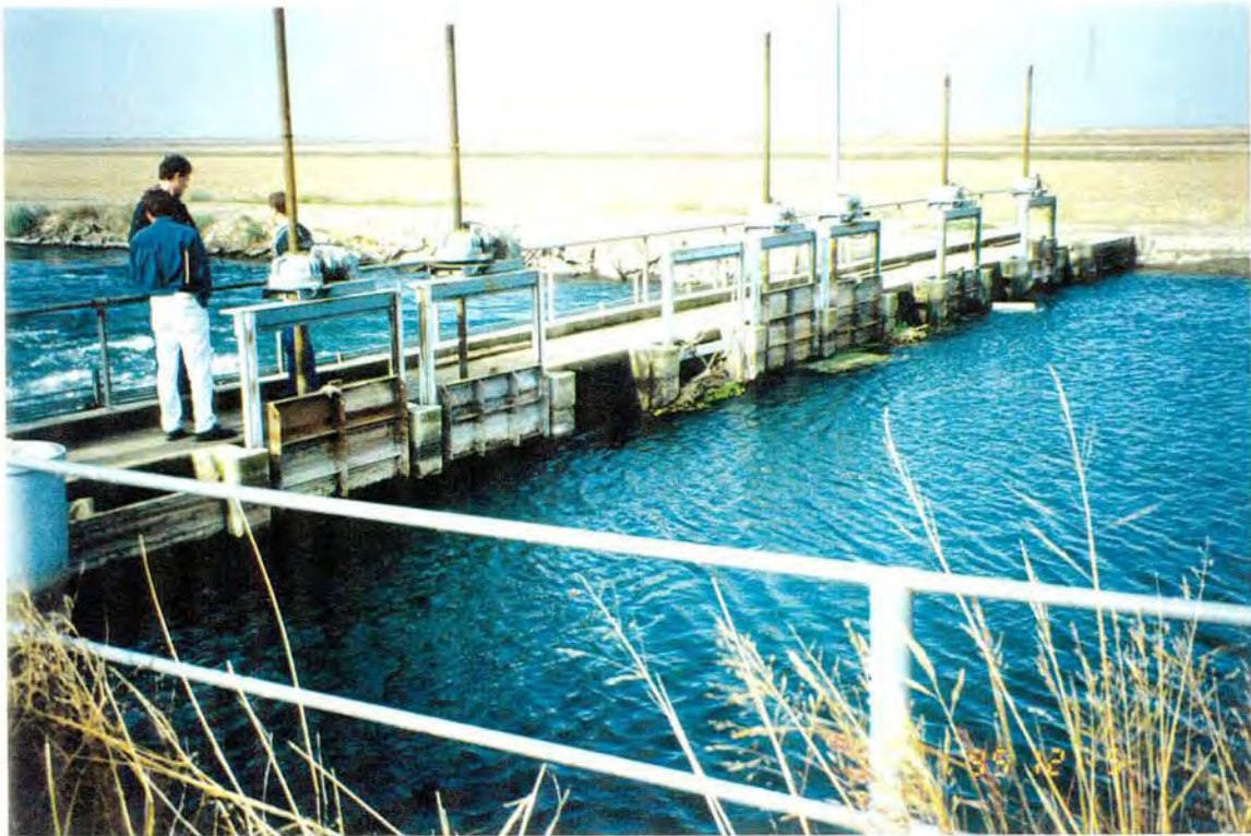
Photograph 8. - Willard check - vertical slide gates in bulkhead slots. Some problems are encountered with binding gates.
