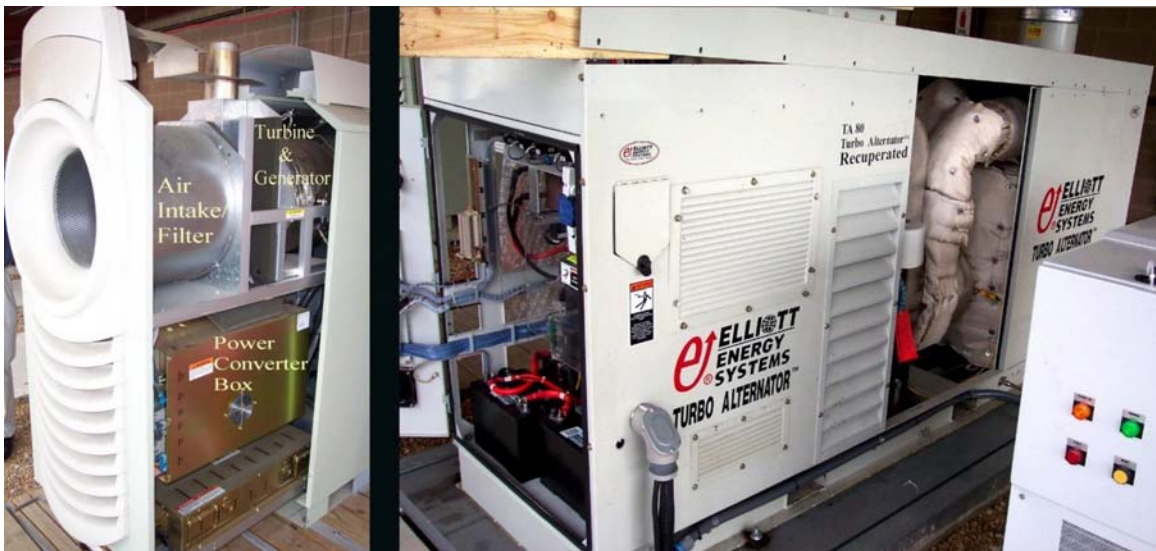
Fig. 3.3. Capstone microturbine (30 kW) and Elliot microturbine (80 kW). Numerous ventilation openings allow ambient air to flow through cabinets.
