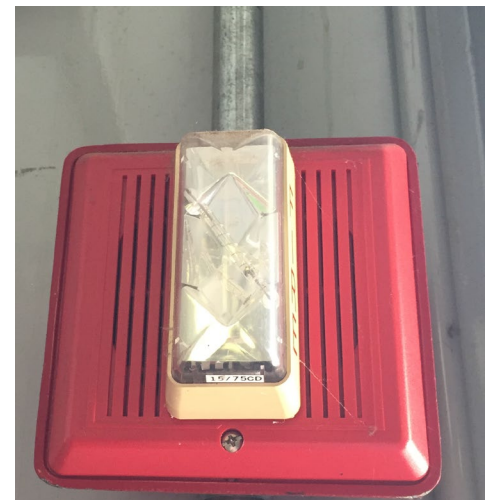
FIRE ALARM STROBES, EXAMPLE OF VISUAL SIGN OF FIRE ALARM
