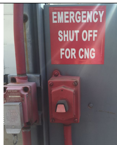
EMERGENCY SHUT-OFF SWITCH
