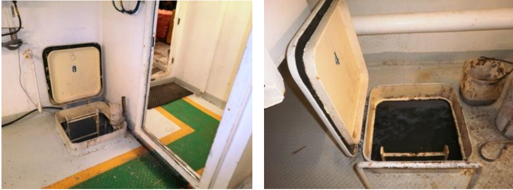
55- Pits in the pit room need solid guards and should not be left open. A tripod should be used for access into the tanks as there is no pad eye above the hatch for attaching any type of fall protection
