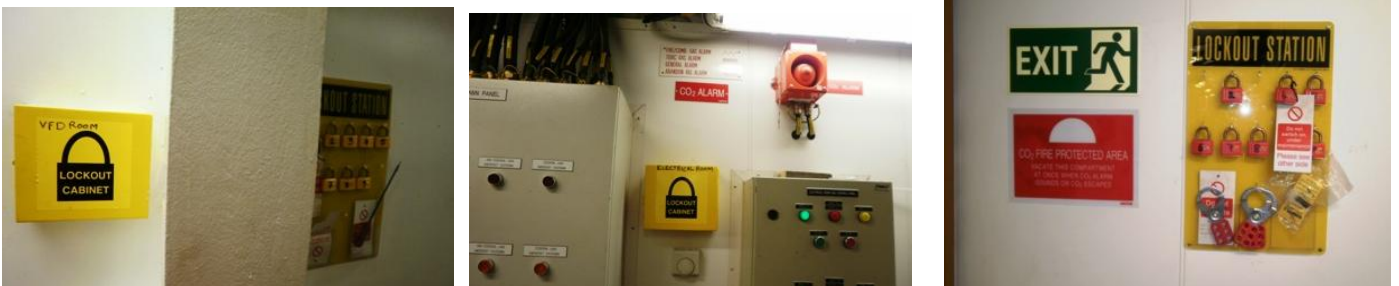
57- Electrical lockouts are not being carried out as per policy. The supervisors need to review the LOTO policy and educate the crew on the same. Crew to review SAF 320.00 and SAF 460.00
