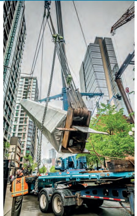
The rigging plan allowed single crane picks where possible and didn't require the use of a tailing device.
