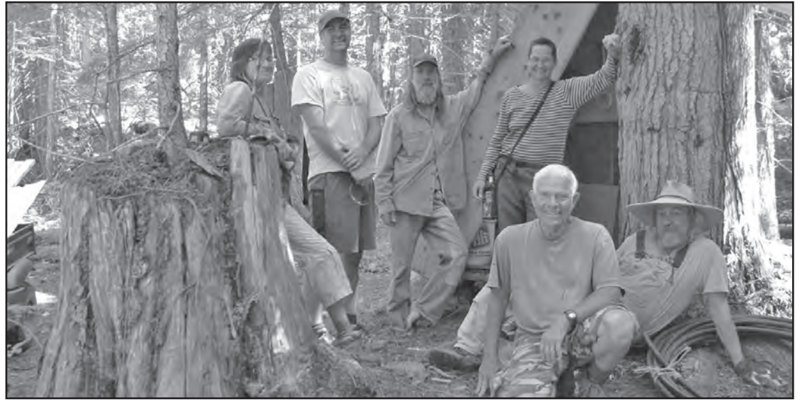
Some of the many volunteers on the epic Johnson's Landing water system project.
