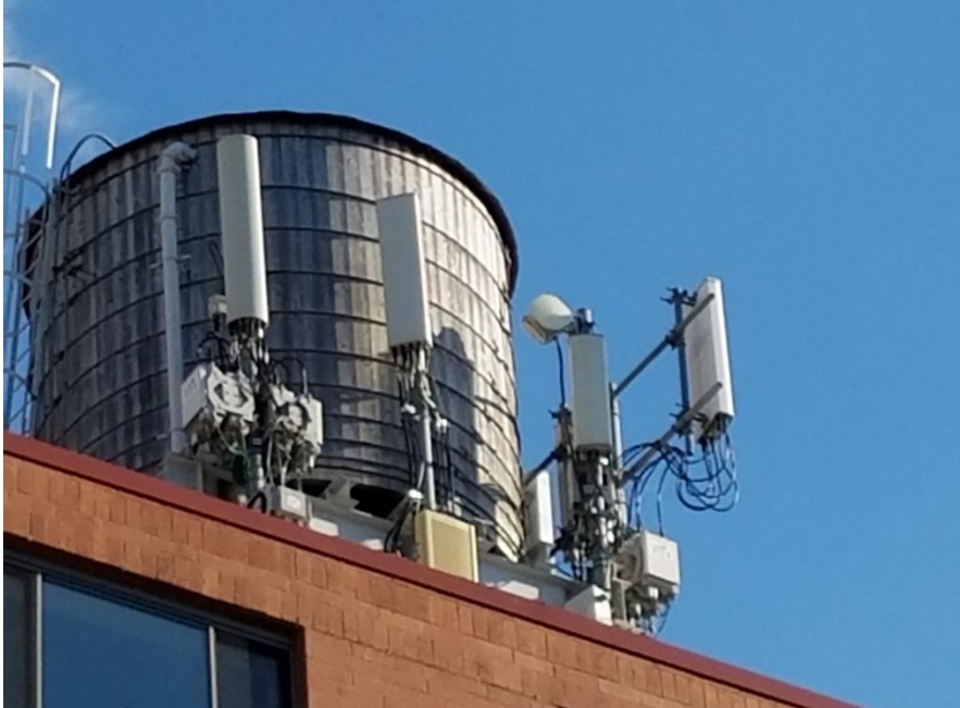
Water Tanks and Telecommunications Cell Sites
