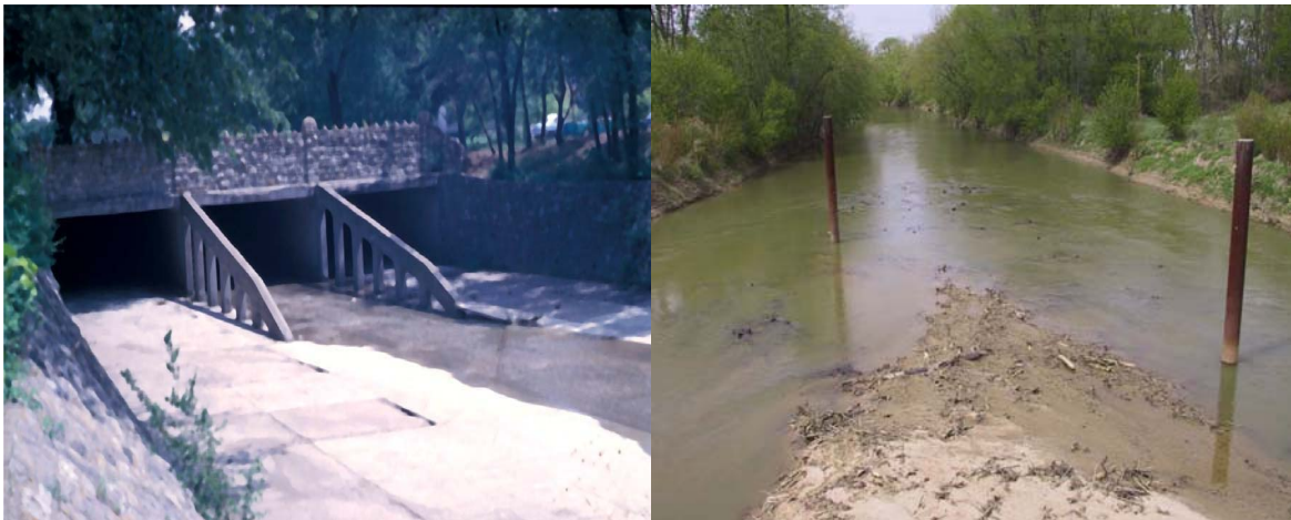
Figure 5: Concrete debris fin extending upstream from bridge pier (left) and debris deflecting posts (right) (Lagasse et al., 2010)
