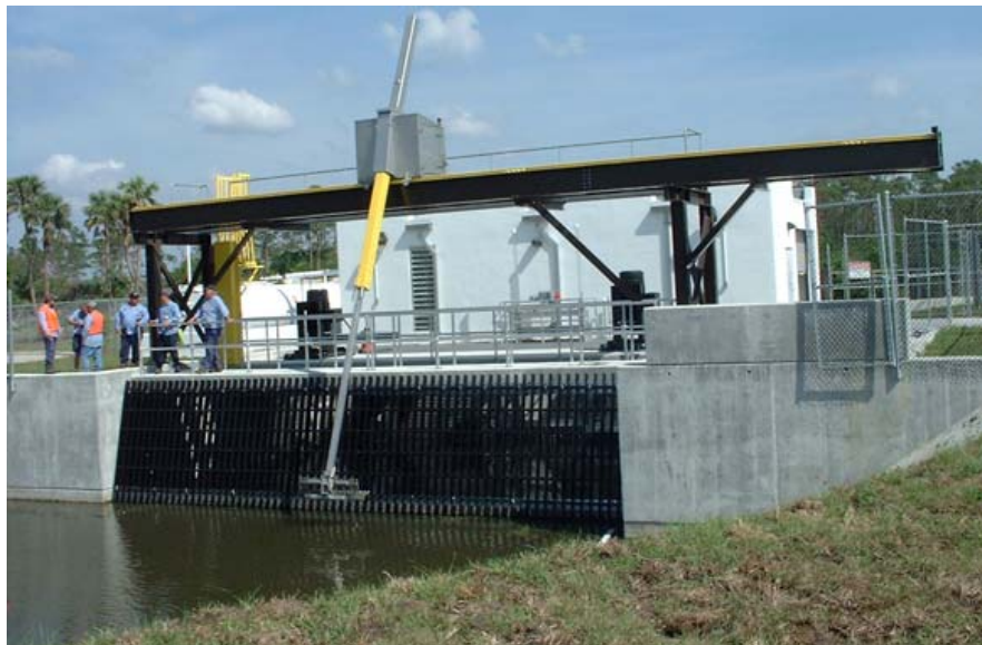
Figure 9: Trash rack and mechanical debris rake (Hydro Component Systems, 2007)
