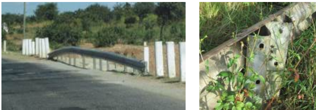
FIGURE 6 Poor guardrail installations: (a) no length of need to hazard or terminals and (b) guardrail used as posts.
