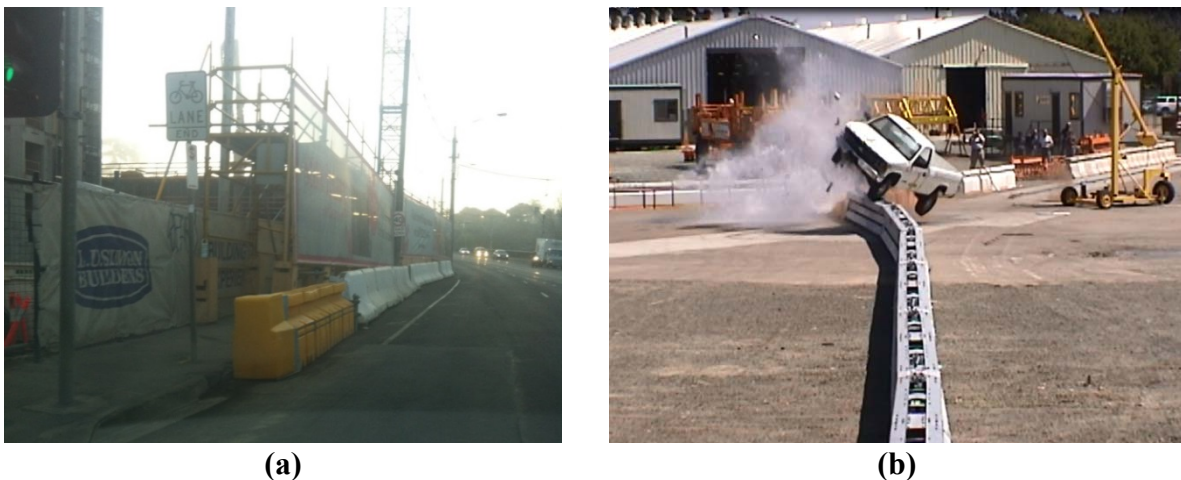
FIGURE 3 Examples of poor installations of temporary barriers: (a) lack of 22.5-m long by 6-m wide run-out area and (b) gating nature of the terminal used in the example.
