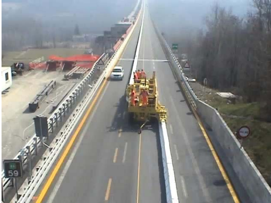
FIGURE 1 Use of a movable barrier to provide tidal flow when an opposing carriageway is being reconstructed.
