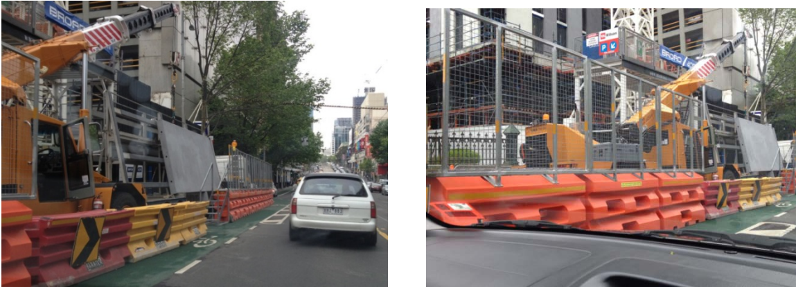
FIGURE 4 Unacceptable use of plastic water-filled devices.
