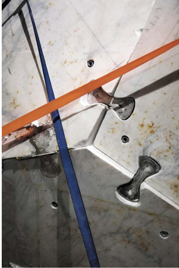
Figure 13. 6-piece mock-up, detail showing unit 3 and 5 locked with the in-situ casting technique, and unit 6 supported by 2 drift-pins.
