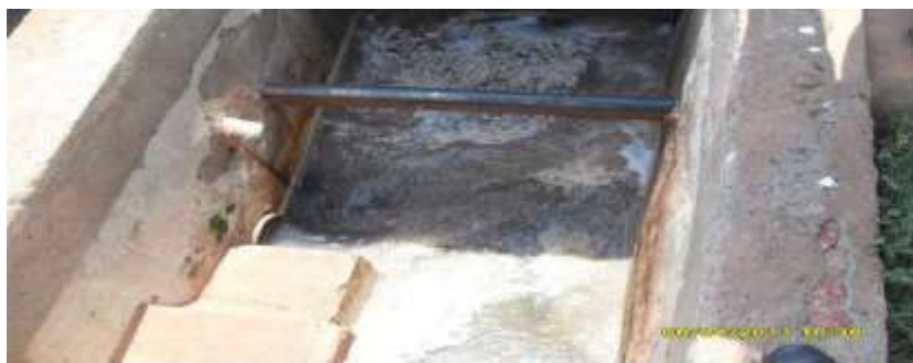
M/s. Gadre Marine Export Pvt. Ltd., Ratnagiri, Flow meter at inlet point not installed
