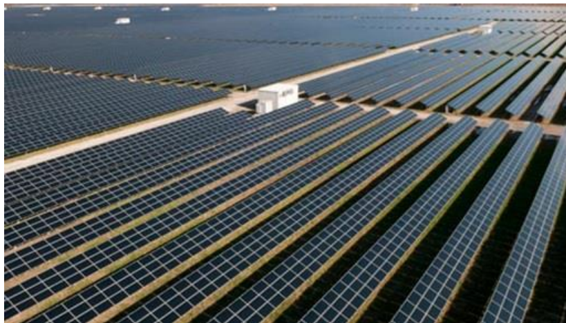
1253 1254 Figure 17 - First Solar, Inc. Solar Cell Array
