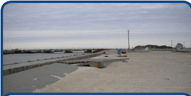
Figure 3: Unrepaired Hurricane Ike damage to Rollover Pass. Photo taken in February 2011.
