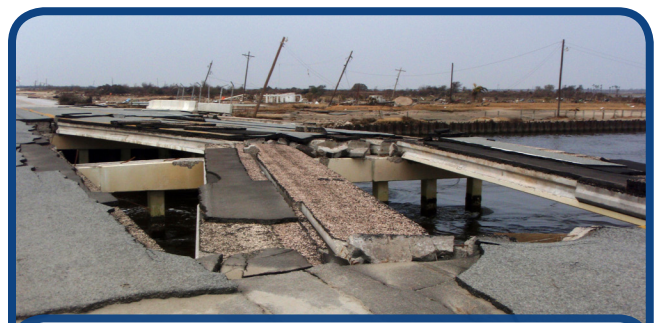
Figure 2: Damage to State Highway 87 bridge over Rollover Pass due to Hurricane Ike. Photo taken in September 2008.
