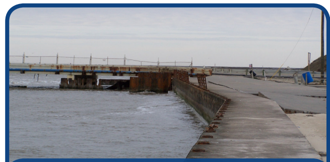
Figure 5: Missing handrail at the southeast quadrant of Rollover Pass. Photo taken February 2011.
