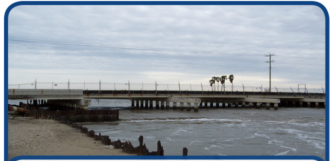
Figure 4: Top of sheet pile at the northeast quadrant of Rollover Pass. Photo taken in February 2011.
