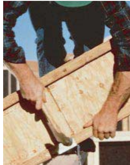
Figure 3. Sloped-seat connectors like the Simpson VPA or the USP TMP can provide bearing at the top plate if the roof loads are not too great.
