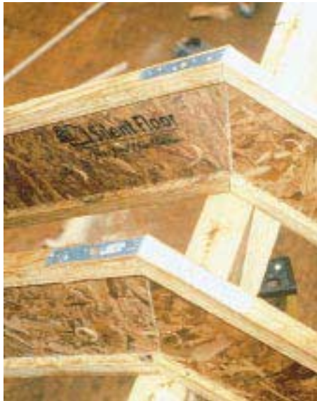
Figure 2. When supporting I-joists on a beveled plate, install metal straps across the tops of the butting joists for all roof slopes. When using hangers, straps are necessary for slopes above 7/12.
