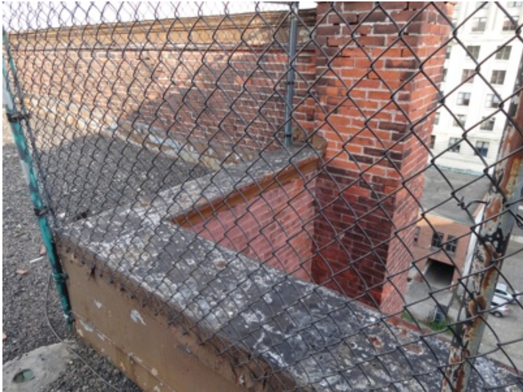
Detail D: Showing the existing condition of the coping, holes in mortar beyond, chain link fence.
