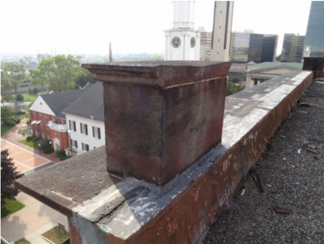
Detail I: Showing the stone cap and the termination attempt of the metal on the back side.
