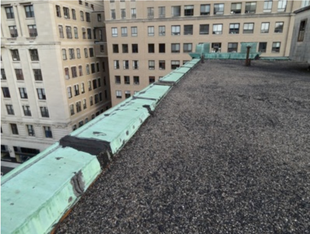
Detail H1: Photos on the left show the interior and exterior views of the copper coping and exterior dental detail.
