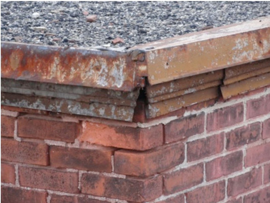
View of the exterior portion of the building showing the distressed coping details and the tuck pointing issues.
