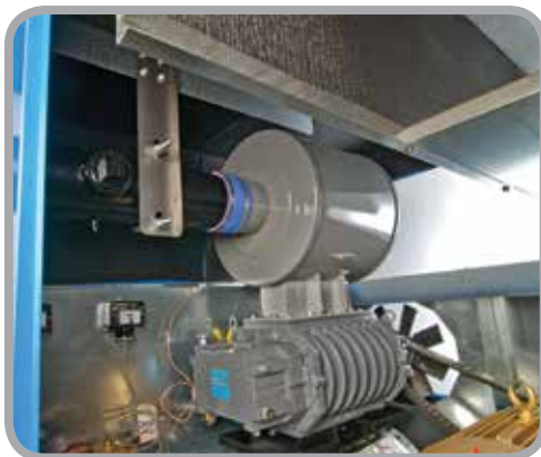
View with rear panels removed
