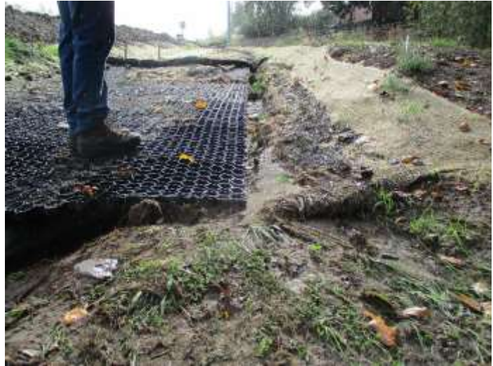
Figure 2-7 Erosion control failure at water quality facility
