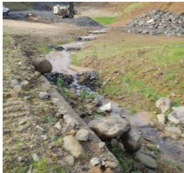
Figure 2-11 Check Dams slow runoff velocity
