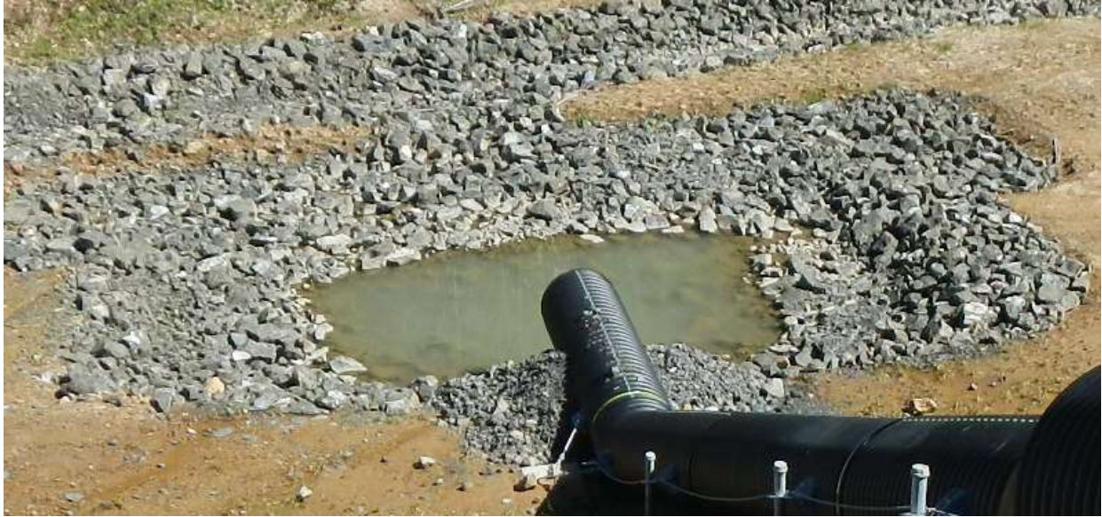
Figure 3-16 Energy Dissipater (permanent installation)
