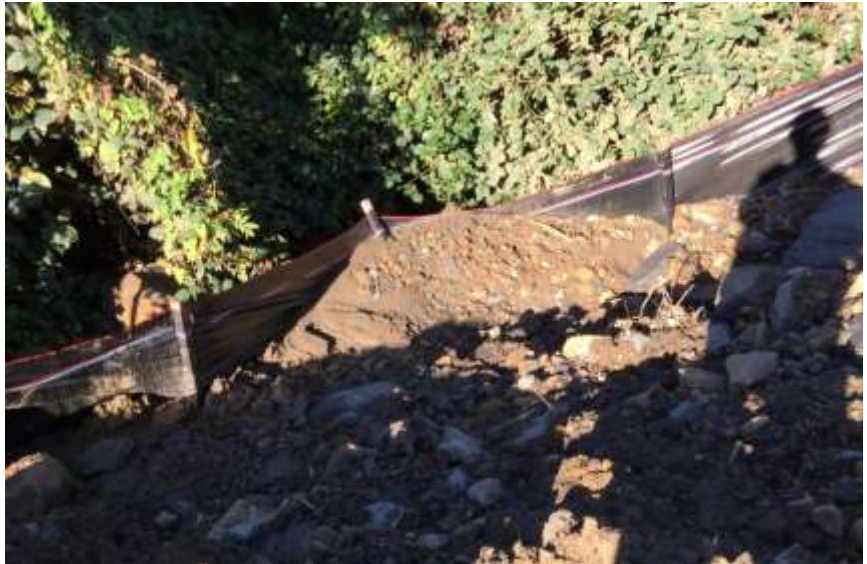
Figure 3-29 Sediment fence maintenance failure
