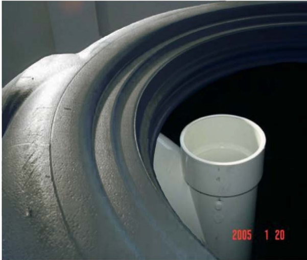
Photo 4.1.16-Pipe located inside the edge of the manway
