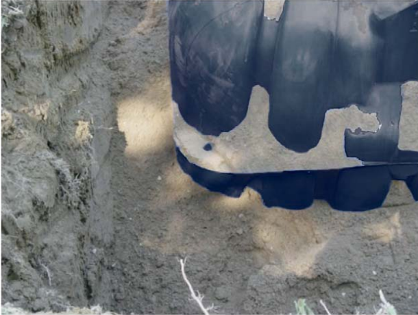
Photo 4.1.7-Proper support for vessel
